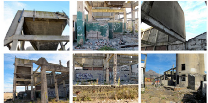
The state of the concrete work on site. One of the biggest issues is spalling
