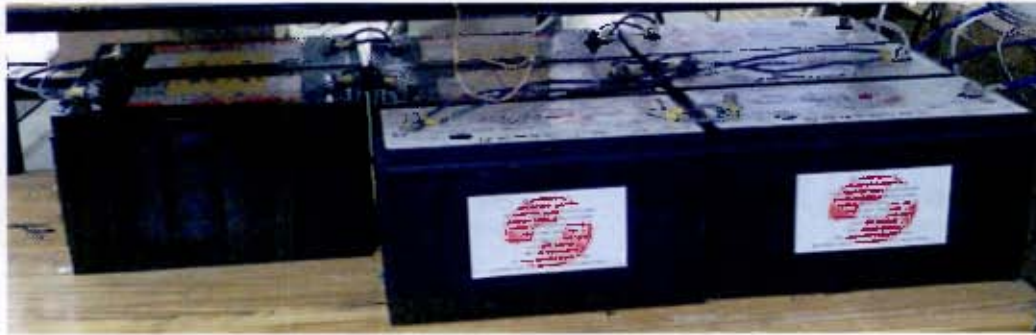
Photo 5.1.3-2: Eight Lead-acid batteries assembled to make 96V dc bus
