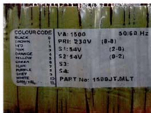
Photo F.1-1:Single-phase three winding transformer information plate
