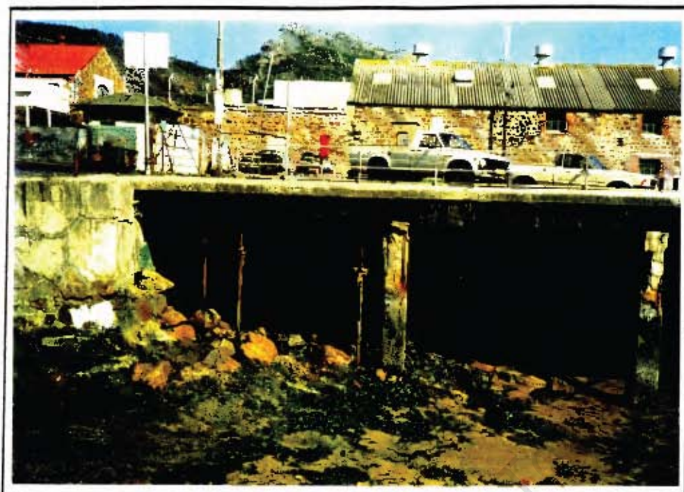
Figure 5.21a: Corrosion Damage of Simonstown Jetty
