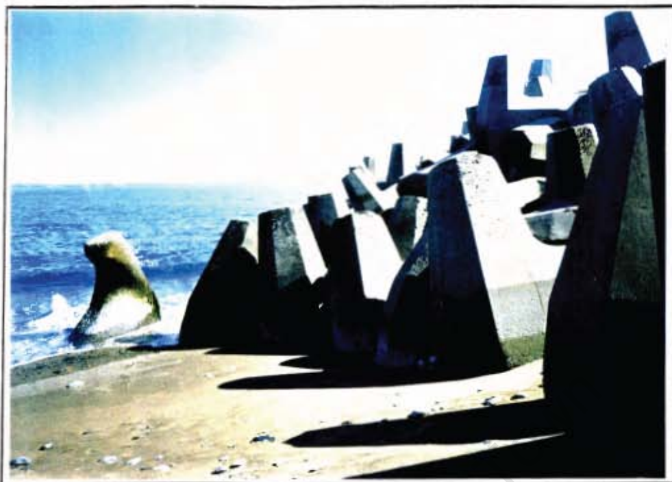
Figure 5.14a: General Condition of Concrete on Dolosse
