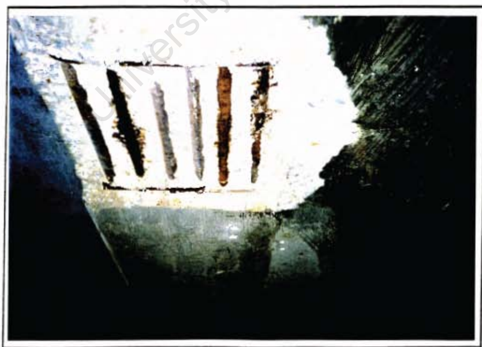
Figure 5.18: Corrosion Damage of Touw River Bridge
