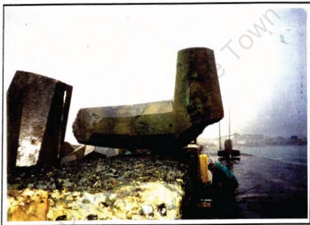
Figure 5.17a: Example of Physical Damage of Dolosse
