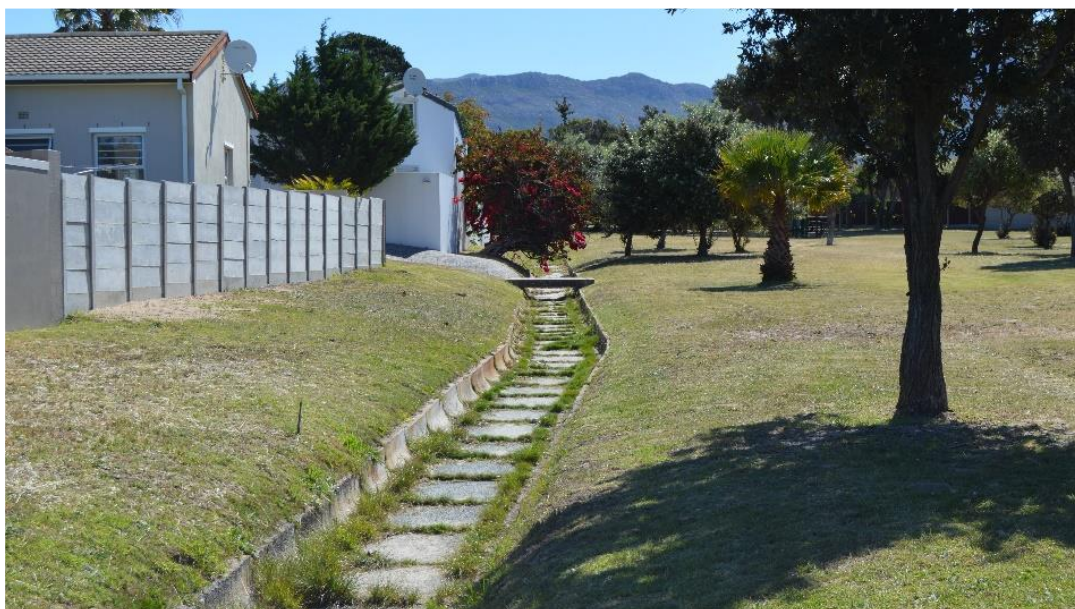
Figure 6-2: Concrete-lined channel with vegetative outgrowth in Westlake, downstream of Klein Wassenaar Road (Source: Geordie Thewlis)
