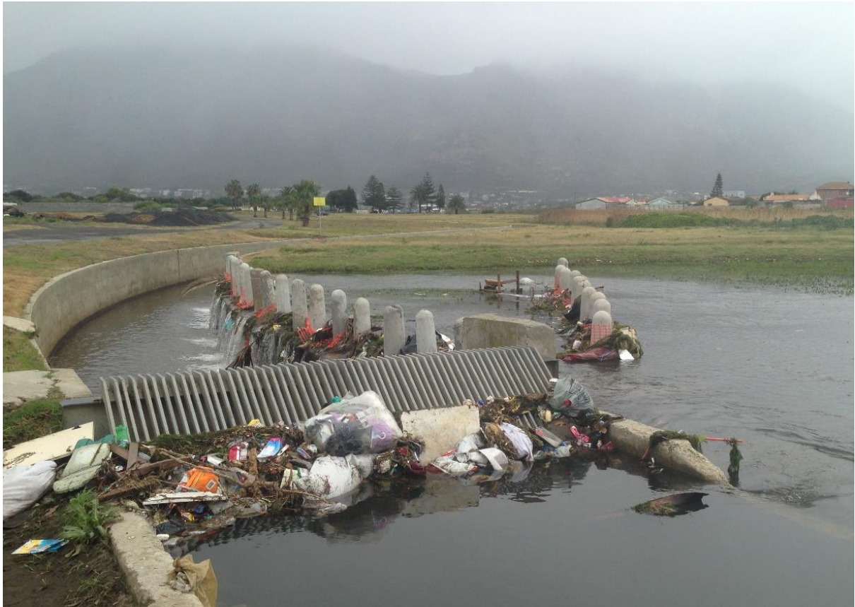
Figure 3-4: Blocked litter trap on the Sand River Canal during a storm
