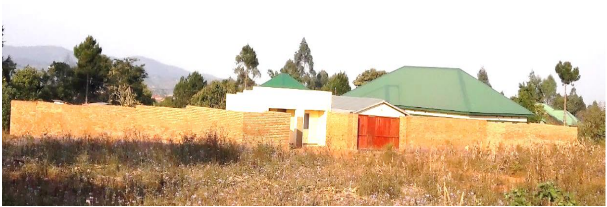
Figure 5.9: Planned House next to ADMARC Regional Manager’s House at Geisha shows the Confidence of Inhabitants
