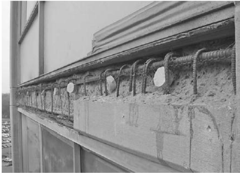
Figure 3.5: Embedded zinc anodes used in concrete rehabilitation to prevent the formation of new corrosion sites adjacent to completed patch repairs (Roberge, 2008)
