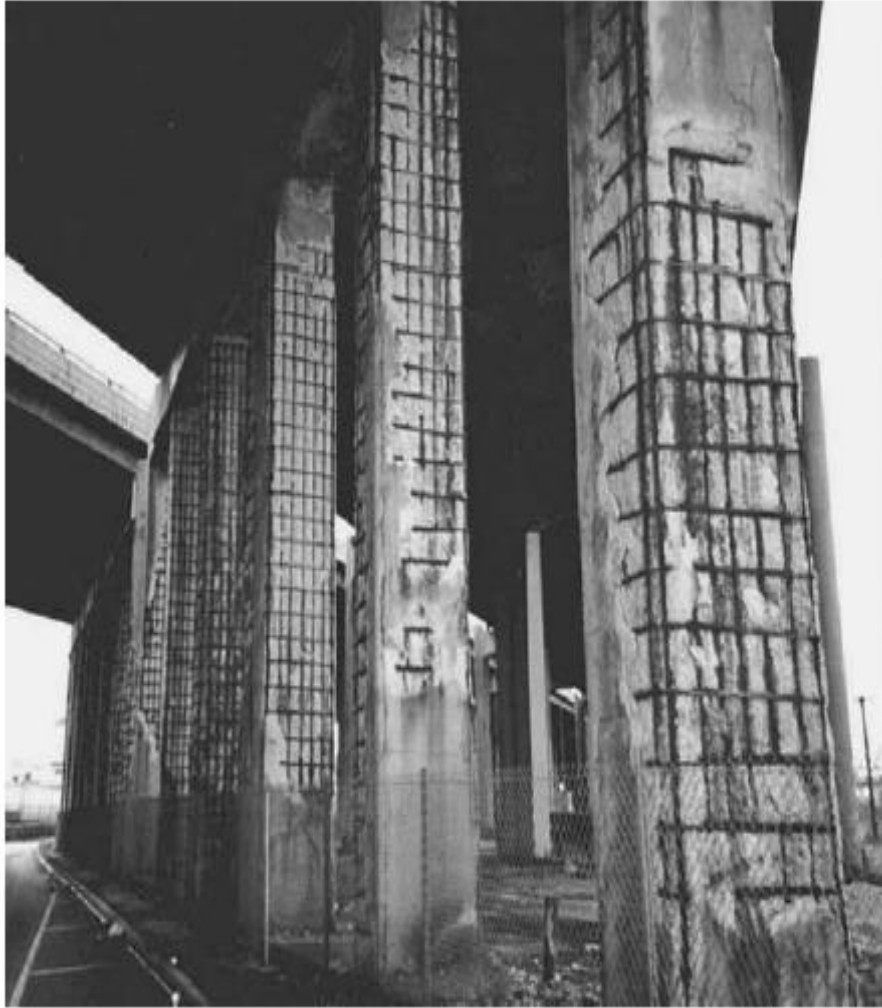
Figure 2.7: Corrosion ravaged columns of a highway bridge in Illinois (Roberge, 2008)
