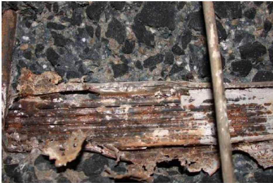
Figure 2.11: Corroding prestressing steels after opening of the duct (Source: http://www.efcweb.org/Working+Parties/WP+11/WP+11+History.html accessed on 18 th November 2011)
