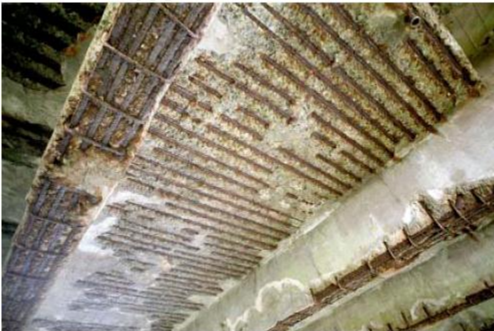
Figure 2.8: Concrete spalling from the underside of a bridge deck (Covino et al. , 2002)
