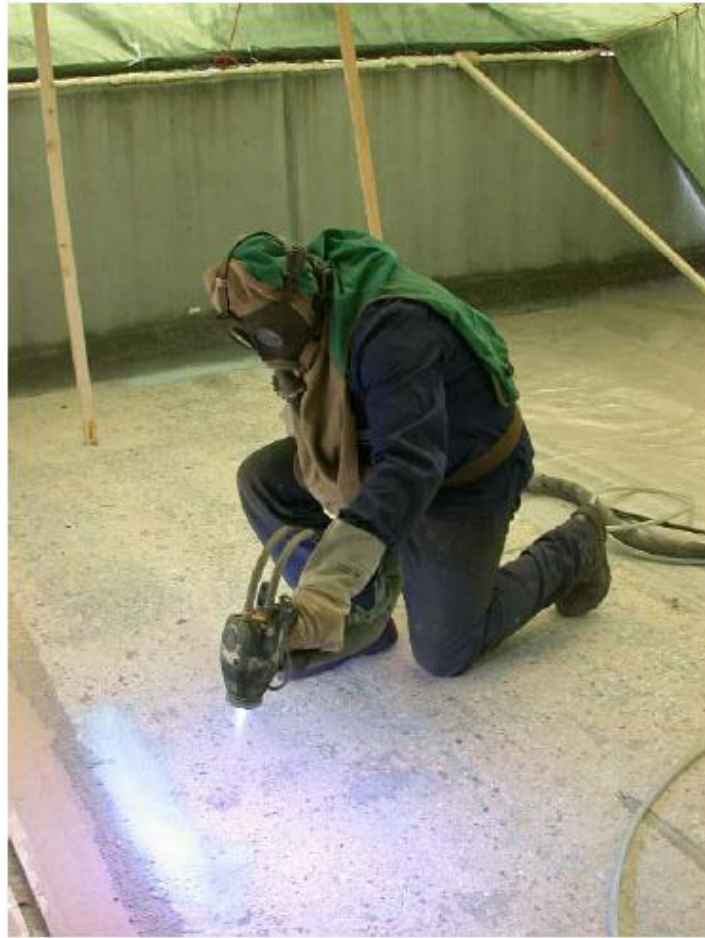
Figure 3.7: Application of thermal sprayed zinc SACP (Source: http://www.efcweb.org/Working+Parties/WP+11/WP+11+History.html accessed on 18 th November 2011)
