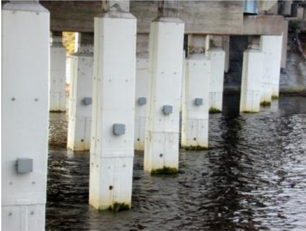
Figure 3.8: Sacrificial zinc jacket around a concrete pile (Source: http://www.pavementpreservation.org/wp-content/uploads/presentations/FDOT%20Cathodic%20Protection%20Practices%20in%20florida.pdf accessed on 22 nd December 2011)
