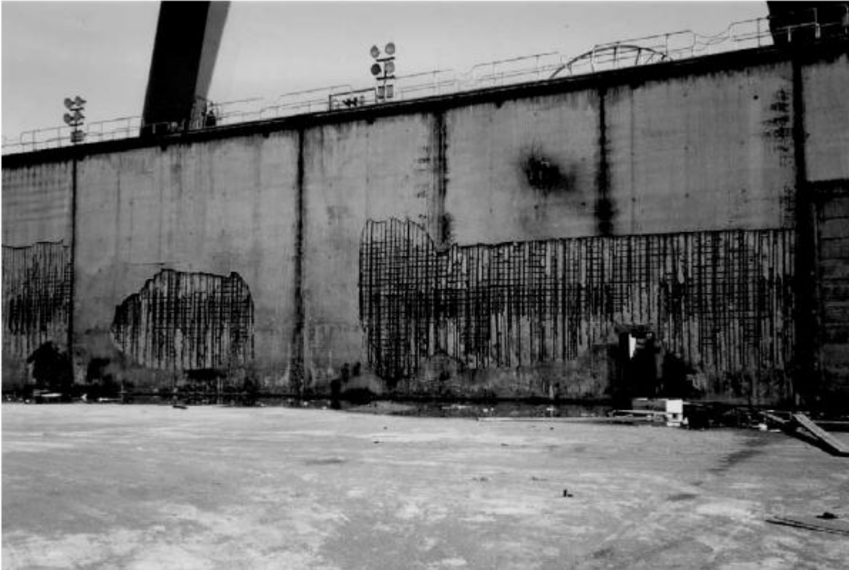
Figure 2.9: Deterioration of a deck wall due to corrosion (Costa and Appleton, 2002)
