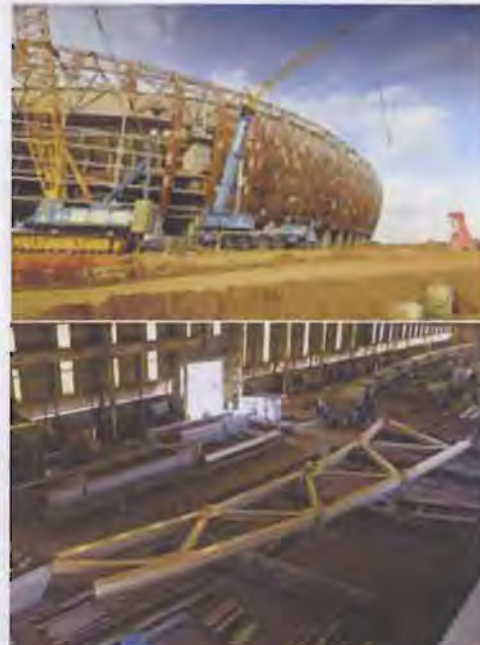
FIGURE 105: Soccer City Stadium, Johannesburg, Boogertman and Partners, 2010 (DSE, 2009) Large prefabricated steel sections were manufactured at a workshop in Vanderbijl Park and transported to site as abnormal loads on large trucks. It shows that the expertise and facilities exist in South Africa for large-scale steel construction.
