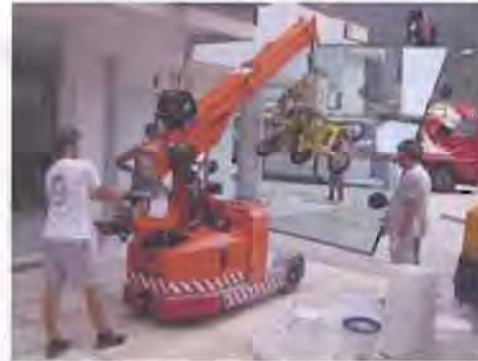
FIGURE 168: Glass Lifting ( www.jekko.it ) The image shows workers operating a small glass lifter.
