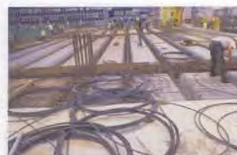
FIGURE 104: 88 Wood Street, London, Richard Rogers, 2001 (Strelitz, 2005) Precast ribs were installed and connected to the structure by post-tensioning. A reinforcing mesh was laid above the ribs and topped with in situ concrete to form the floor surface
