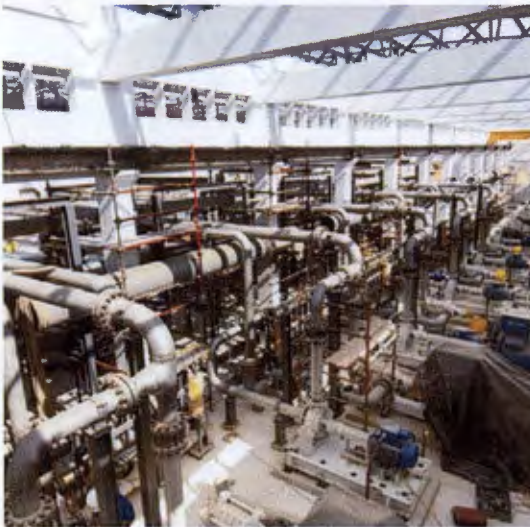
Areva's RO desalination plant at Wlotzkasbaken
