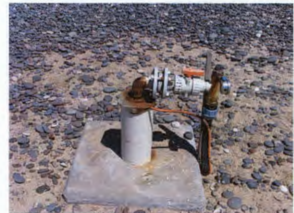
Mowe Bay: Elements of the small scale reverse-osmosis desalination plant Images: G Howard
