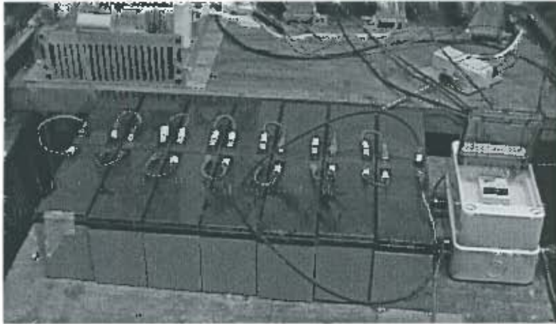
Figure 6-14. UPS Battery Set
