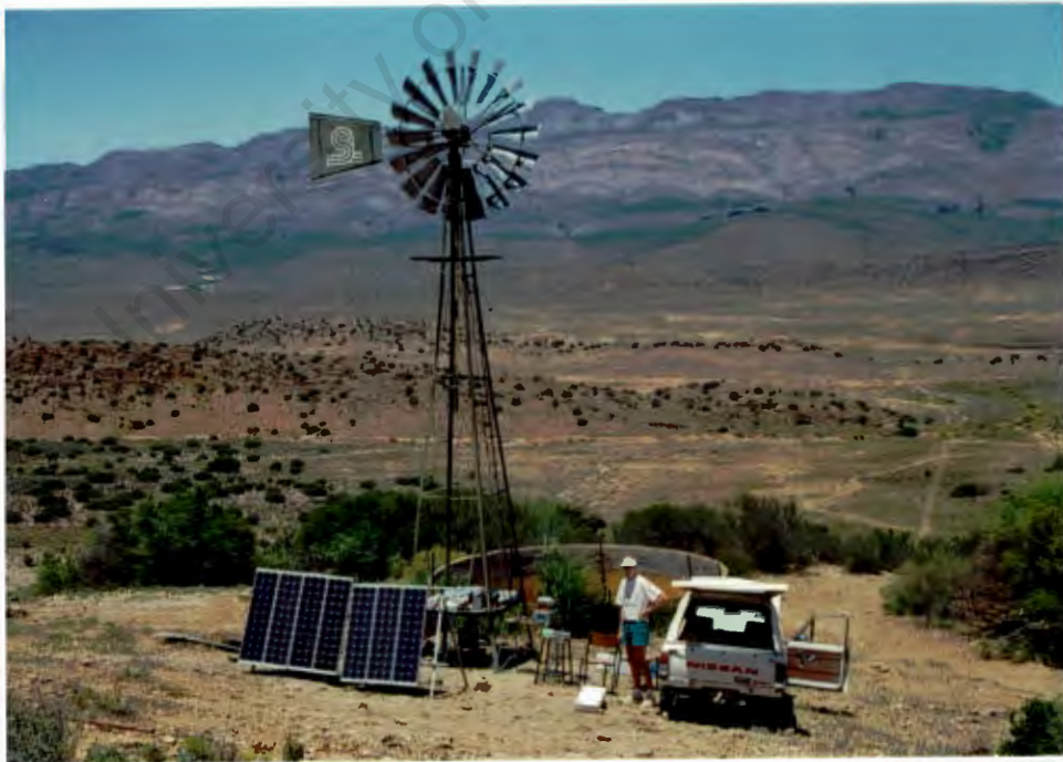
Figure 58: The Borehole Pump Used for the Field Tests
