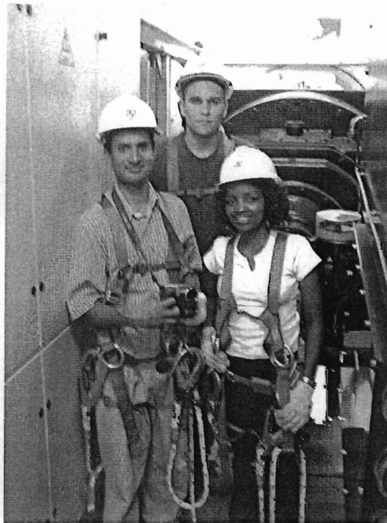
Figure 3. 2 Inside V66 Nacelle, with generator at the background
