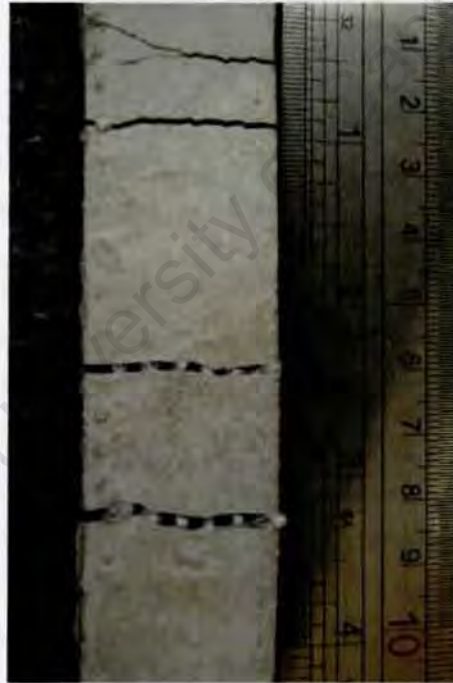
Figure 5.45: Typical very fine cracks on a post-loaded sample (scale on the extreme right is in cm and mm)
