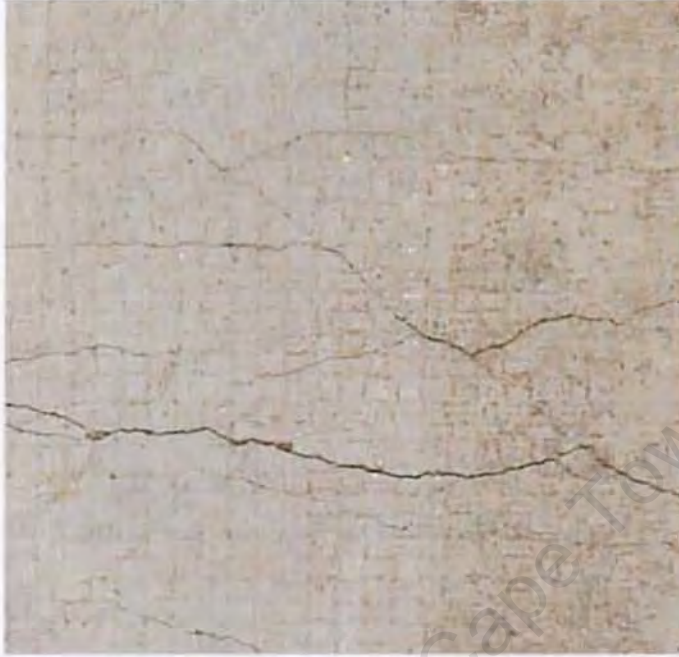
Figure A.2: Multiple cracks after specimen failure
