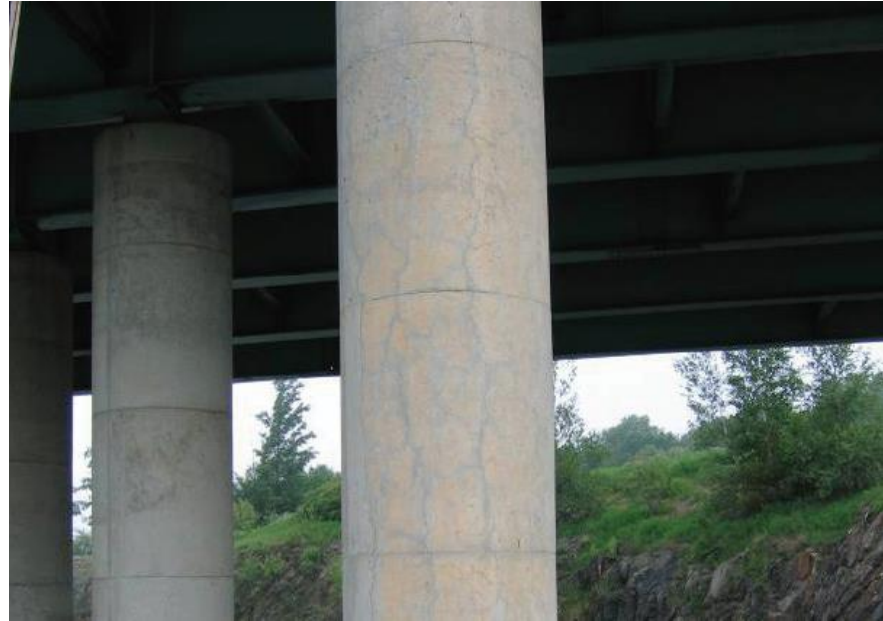
Figure 2.6: Preferred alignment of cracks in an ASR-affected concrete column (US Department of Transportation, 2012)
