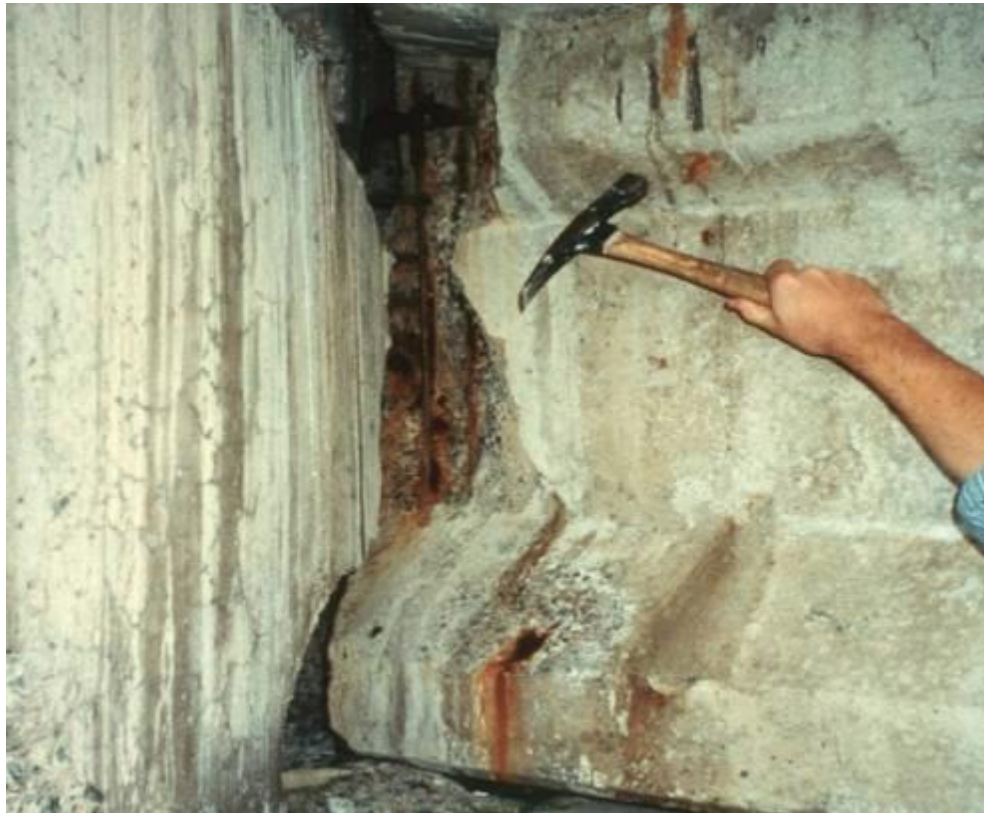
Figure 2.9: Expansion of bridge girder leading to loss of clearance between the girder and embankment and eventual crushing of girder (US Department of Transportation, 2012)
