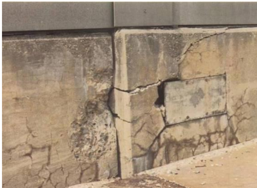
Figure 2.7 Relative movement of abutting sections of parapet wall in a bridge structure (US Department of Transportation, 2012)
