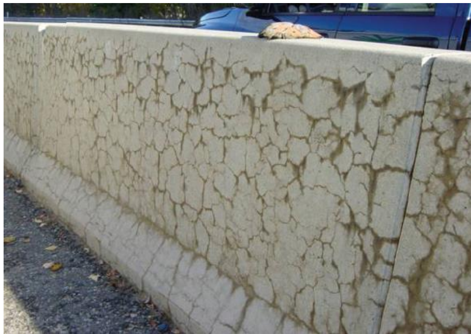
Figure 2.5: Map cracking and associated gel staining around cracks in a median highway barrier affected by ASR (US Department of Transportation, 2012)
