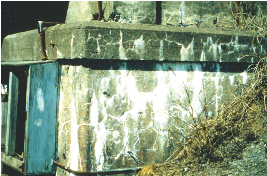
Figure 2.4: Efflorescence and exudations of ASR at the surface of a 25 year old highway bridge concrete foundation (US Department of Transportation, 2012)
