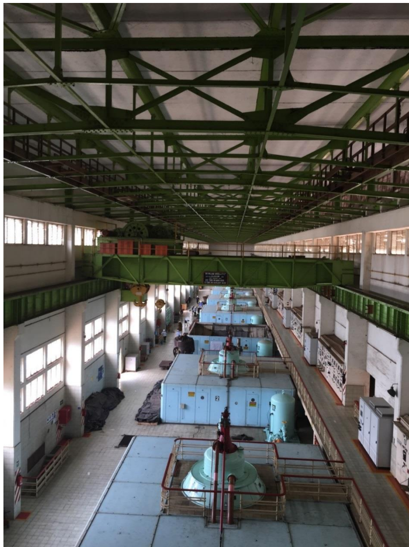
Figure 3.3: View down the Generator Housing Hall
