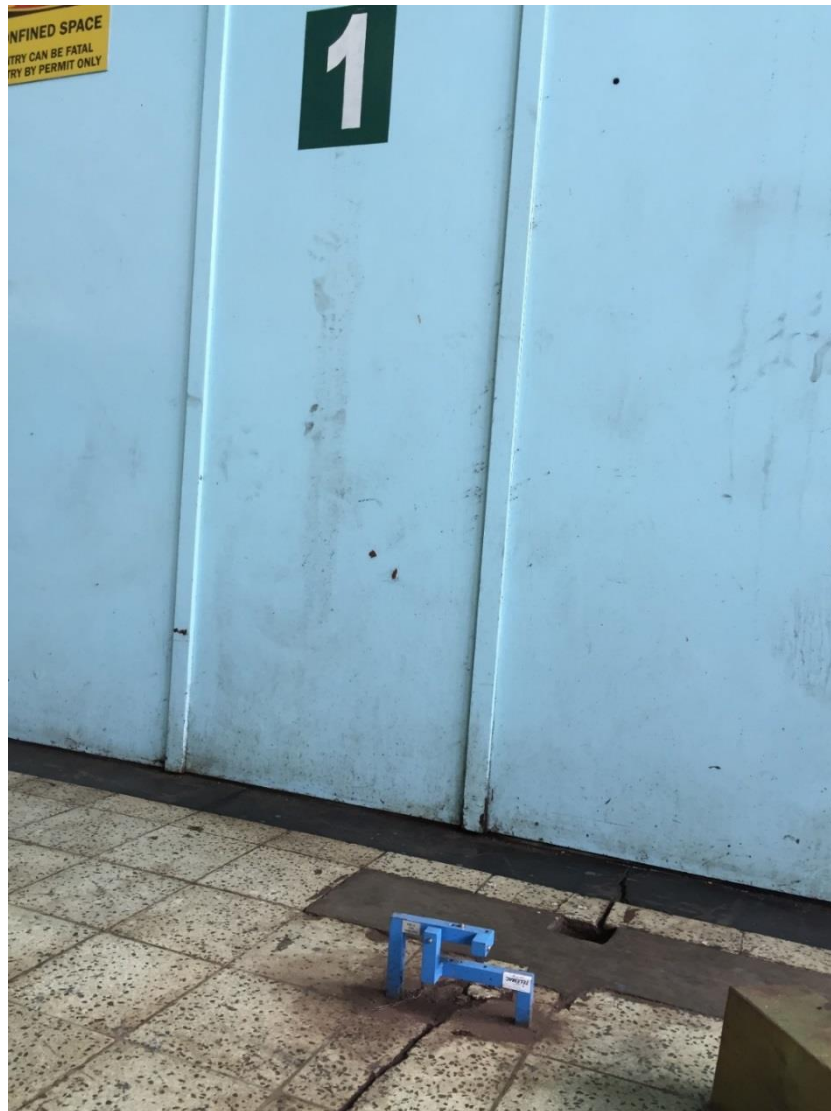
Figure 3.4: View of the longitudinal crack in the machine hall floor
