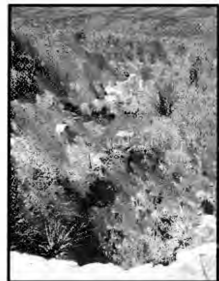
Plate 11 and 12: Site 6 (Stokoe River) a tributary of the Palmiet River, situated within the Kogelberg Nature Reserve. Picture 11 taken mid-stream looking upstream. The presence of a semi-dirt/cement road forces the stream flow through a 50cm cement culvert (seen at the top-middle within this photo), located beneath the road. Photo 12 taken from dirt/cement road, looking downstream. Site code: SR.
