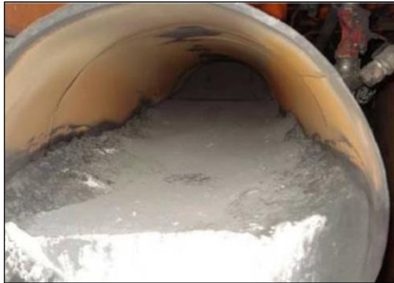
Figure 1-4 – A clogged pipe due to PC settling at a power station, taken from Van der Merwe (2014)
