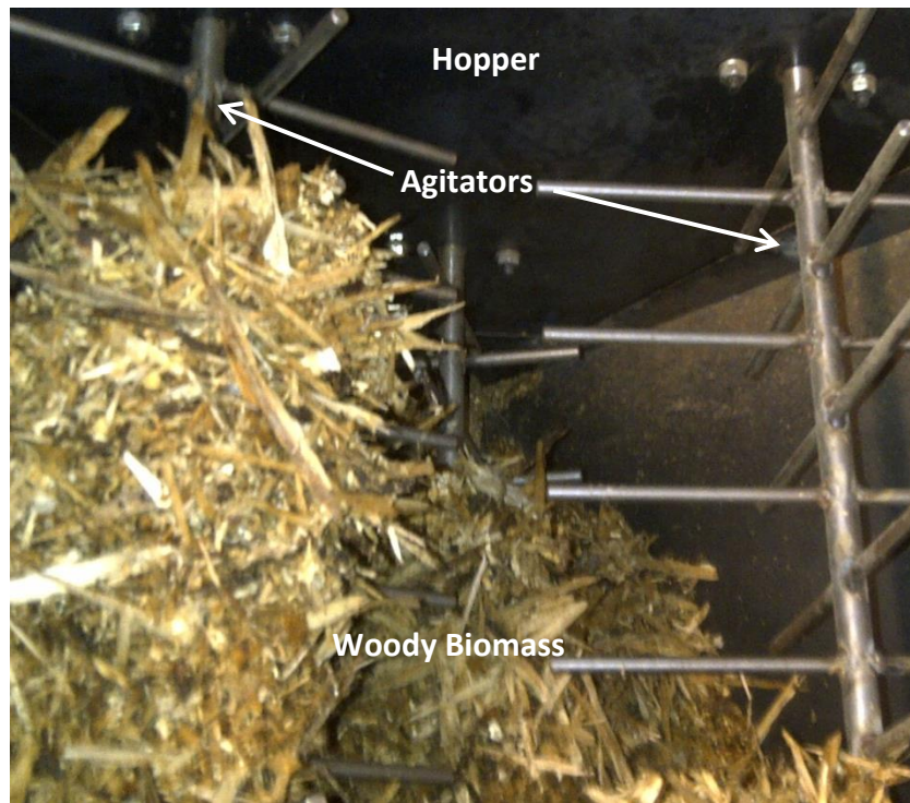
Figure 11.2: Photo of agitators inside the hopper
