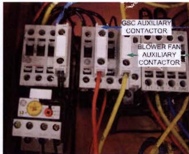
Figure 5.5: Re-wiring the blower fan starter via an auxiliary contact on the soft starter.
