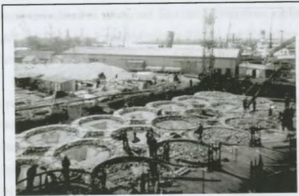
Figure 52 Cape Town: construction of the storage annexe. 31 July 1923. [Port Engineer, Table Bay Harbour]
