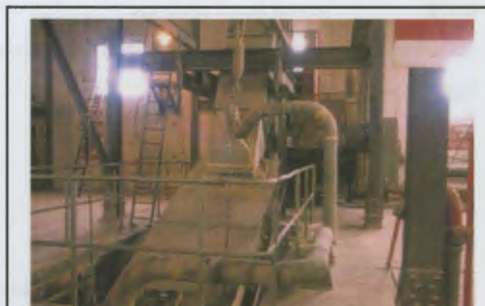
B014: maize chute from elevator head to pre-weigher floor.
