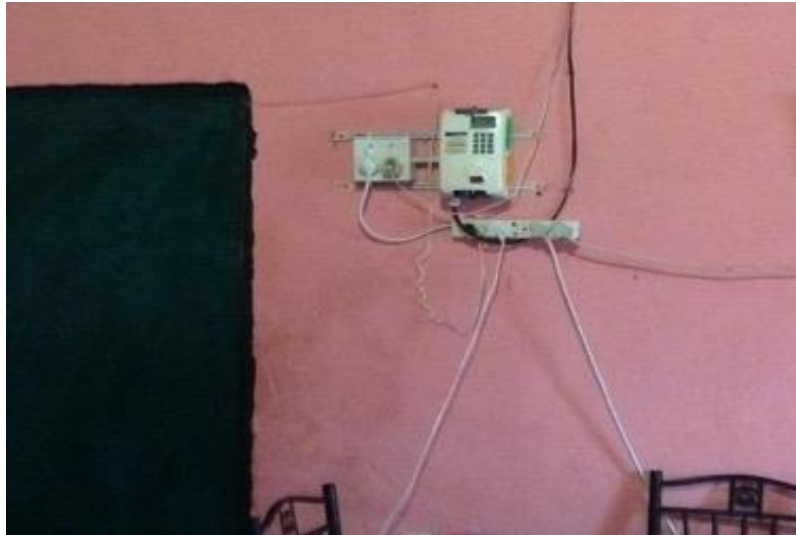
Figure 18: An electricity meter in a house in Snyklip. (Photo by the author, 2016)
