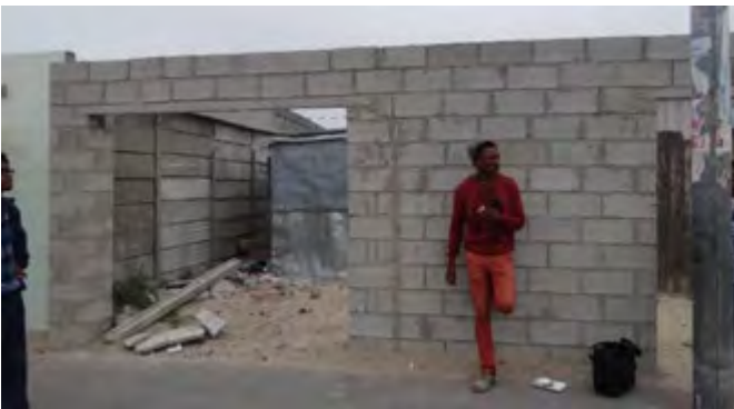
Figure 94 & 95: Two lightweight structures are occupied while a new concrete block building is slowly constructed around the original structure.
