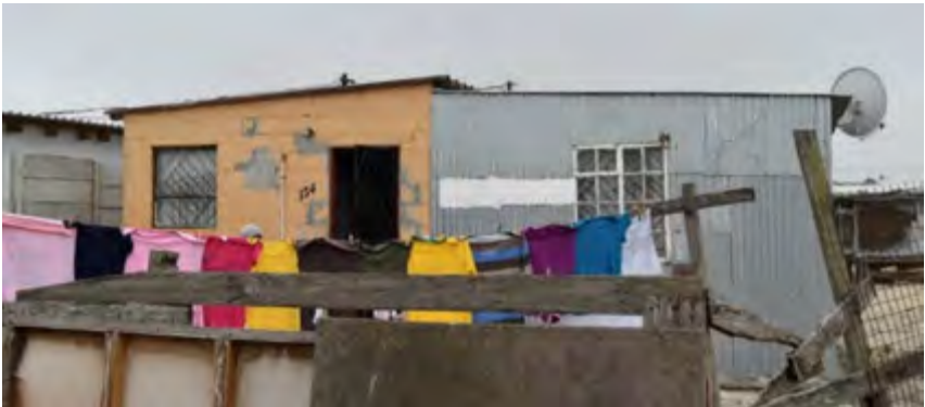
Figure 92 & 93: These two homes have been renovated using corrugated metal along the sides of the houses that are made out of asbestos. The front facades were built out of blockwork.
