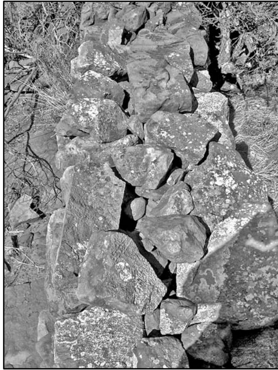
Figure 38: Photograph showing the technique used in the construction of walling at homesteads KS-145 to KS-150.
