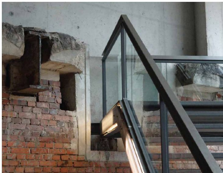
[fig28] Image showing Domenig's approach to 'scab' as manifested in the insertion of a new stair into an existing wall. Existing layers are cut back in order to allow the new to lay claim to space within the oppressive spatialities of the old. [Source: Handa, 2018]
