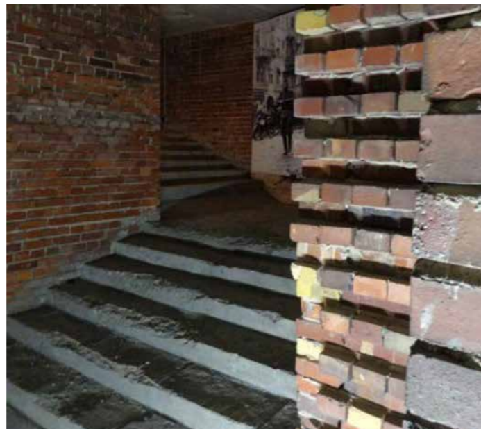
[fig35] Image depicting the protruding brick layers of the existing walls of the Congress Hall which were used to create a spatial and material interaction between the curated materials, the existing architecture, and the viewer. [Source: Handa, 2017]
