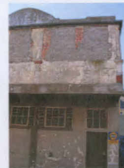
View of building linked to CPUT Student Residence, where the upper floor balcony has been enclosed and openings bricked up
