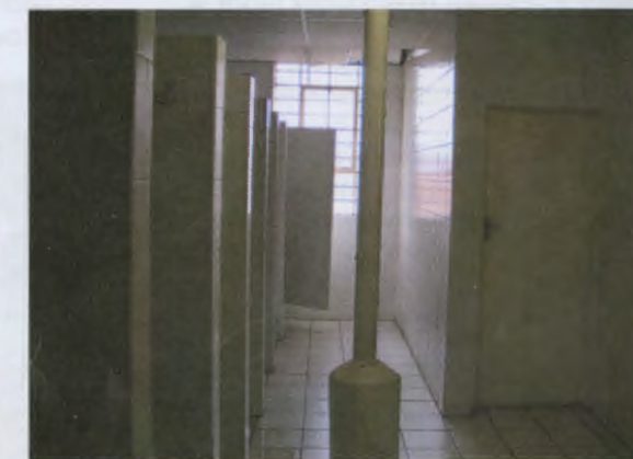
View into new bathrooms. An existing column stands in the middle of the space.
