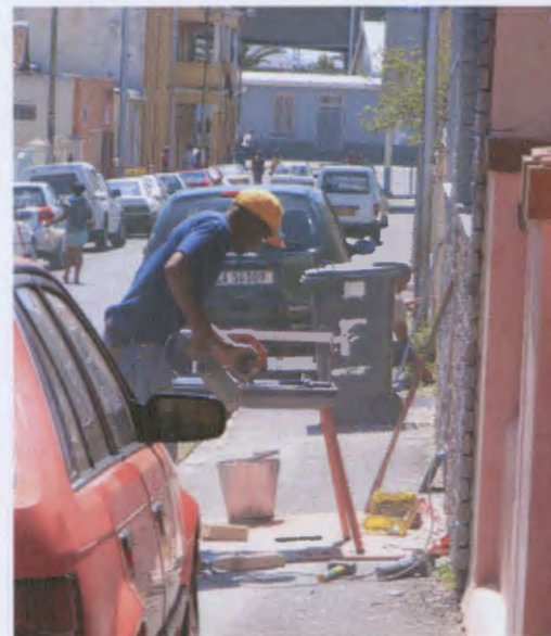
View down Portland Road Here on of Sollie's employees is using the sidewalk as a work area.
