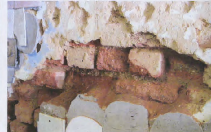
Image showing the current decay of the building. The walls are literally crumbling
