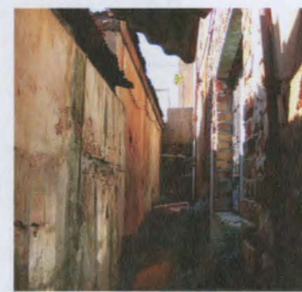
View of Lane 3 looking towards London Road It is covered and used as a storage space
