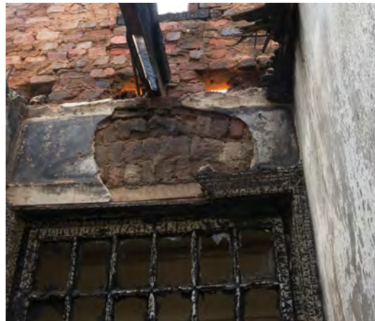
The fire at Montrose exposed brick arches as well as a palimpsest of old and newer infill bricks
