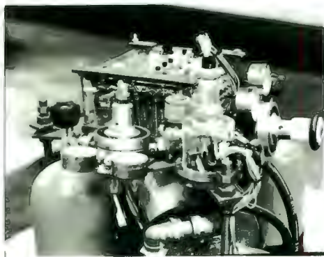
Plate 4.11 Junction Box and Solenoid Valve
