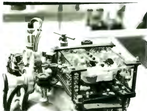
Plate 4.10 Control Box and Air Regulators
