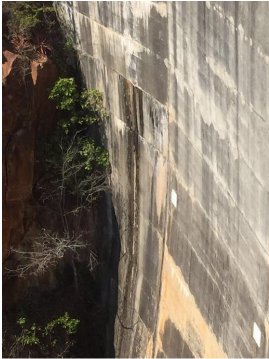
Figure 6-5: View of the horizontal lift joint that displays active seepage
