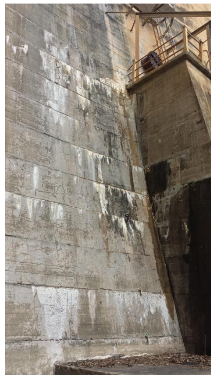
Figure 5-13: Poortjieskloof Dam: Increased cracking in the area surrounding the outlet structure
