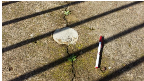
Figure 4-5: Hartbeeskuil Dam: An indication of the crack width and previous core drill hole that determined the depth of the crack
