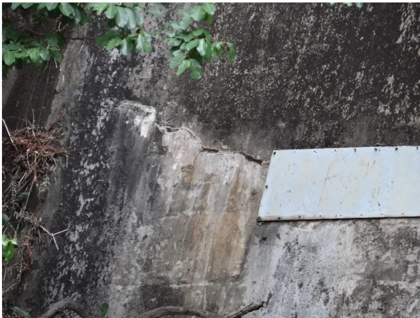
Figure 6-4: The prominent crack near the base of the right flank abutment area
