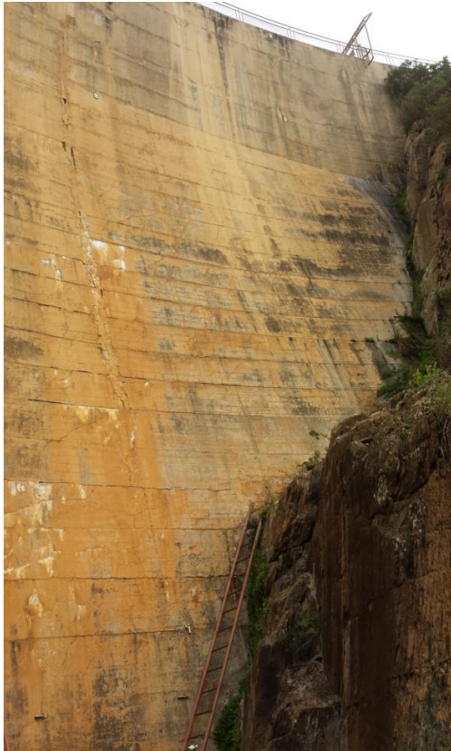
Figure 5-7: Poortjieskloof Dam: Clear parallel peripheral cracking patterns visible on the left flank downstream face
