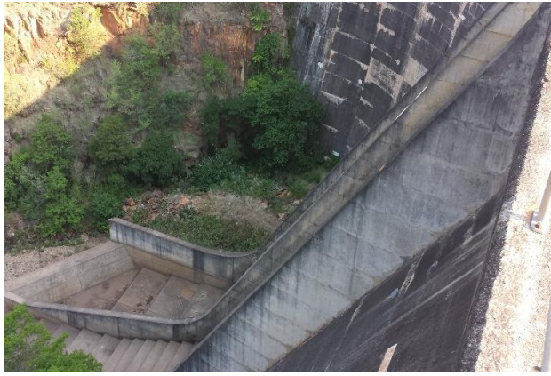
Figure 6-2: The right flank downstream face as viewed from the right flank NOC
