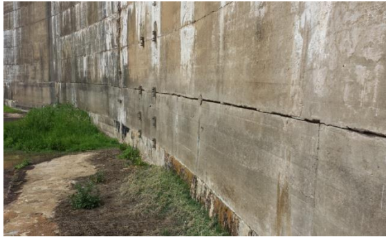
Figure 2-14: Typical separation of a horizontal construction lift joint at Poortjieskloof Dam in South Africa
