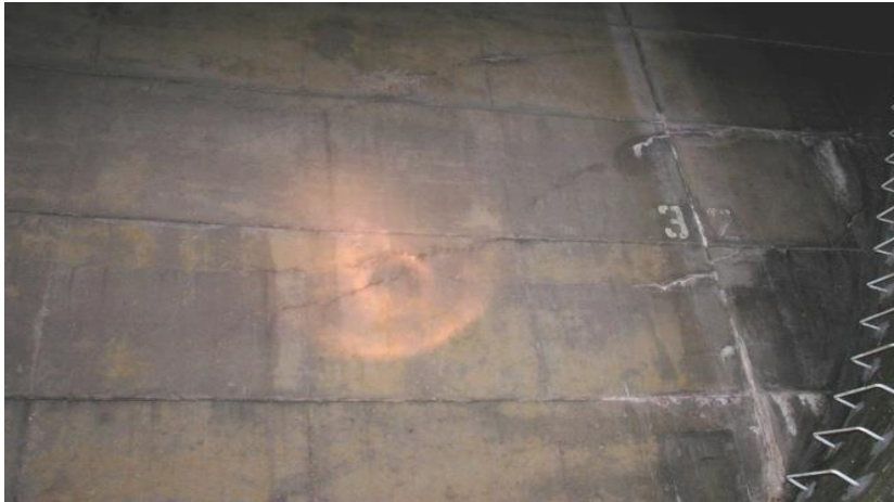
Figure 4-17: Hartebeeskuil Dam: Typical peripheral cracks on the left flank
