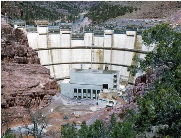
Figure 2-8: The construction of Flaming Gorge Dam in the United States of America (USA) (USBR, 2017)
