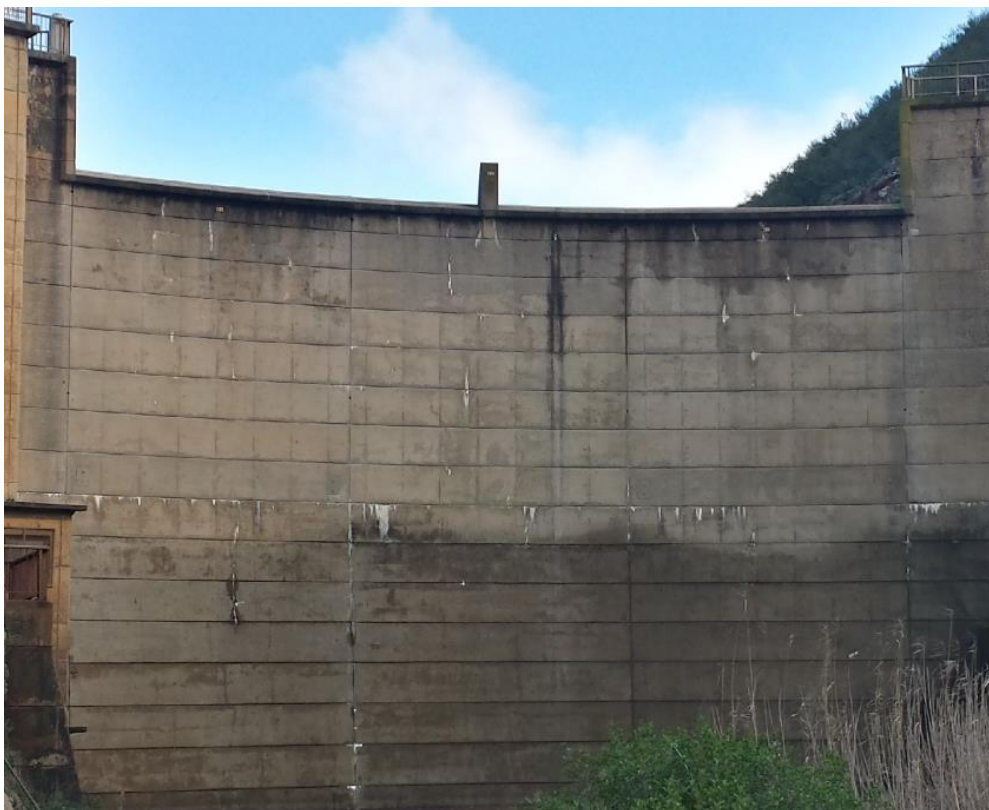
Figure 4-14: Hartebeeskuil Dam: Calcite staining visible on the downstream face of the spillway section
