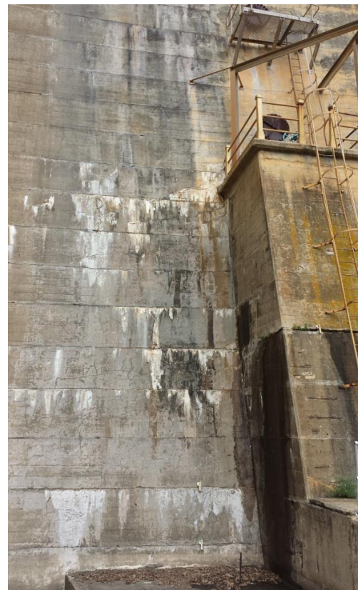
Figure 5-10: Poortjieskloof Dam: Excessive map cracking patterns surrounding the outlet structure; also, note the staining
