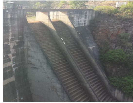
Figure 6-3: The stepped downstream profile of the spillway as viewed from the left flank NOC
