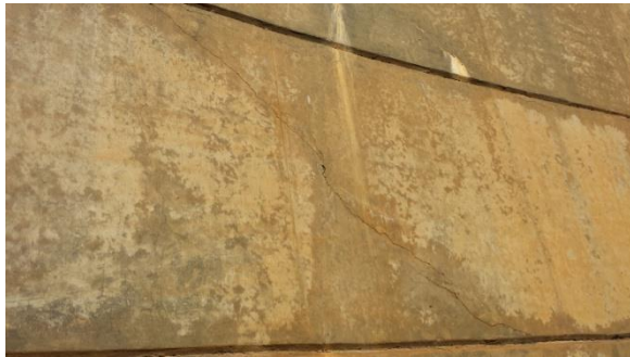
Figure 4-10: Hartebeeskuil Dam: Close-up view of one of the peripheral cracks on the right flank downstream face
