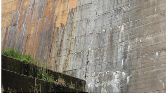
Figure 5-15: Poortjieskloof Dam: Unfavourable cracking patterns on the right flank
