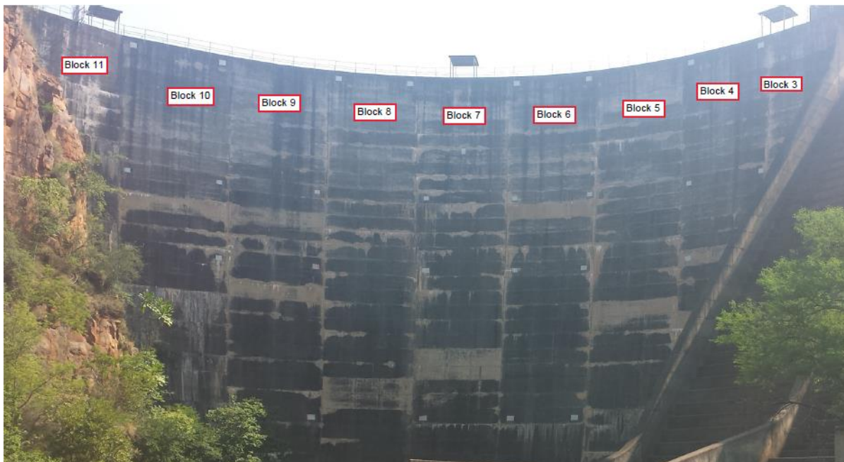
Figure 6-7: The positions of the blocks comprising the arch section at Thabina Dam
