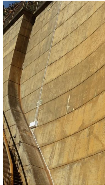
Figure 4-9: Hartebeeskuil Dam: Parallel cracks evident on the right flank downstream face
