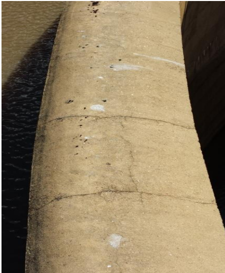
Figure 4-12: Hartebeeskuil Dam: Tangential crack between two radial cracks on the spillway crest
