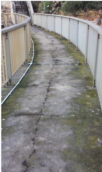
Figure 4-4: Hartbeeskuil Dam: A major tangential crack on the right flank crest
