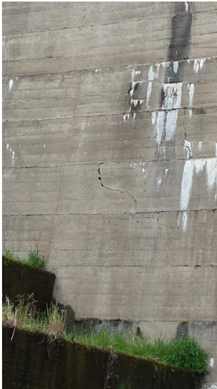
Figure 5-17: Poortjieskloof Dam: A prominent crack parallel to the abutment
