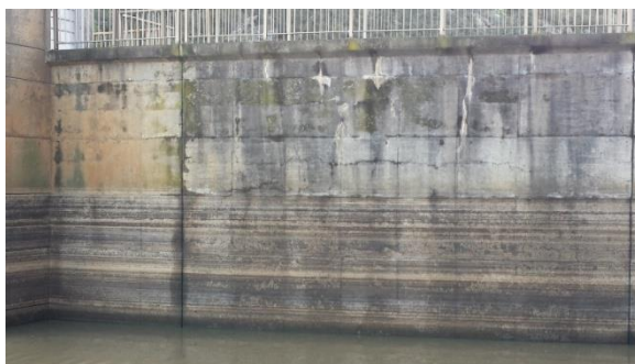
Figure 4-2: Hartebeeskuil Dam: The upstream concrete face of the right flank displaying horizontal cracks
