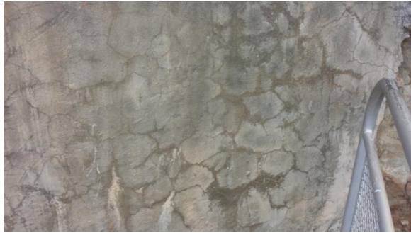
Figure 5-4: Poortjieskloof Dam: Map cracking on concrete step structure left of the NOC
