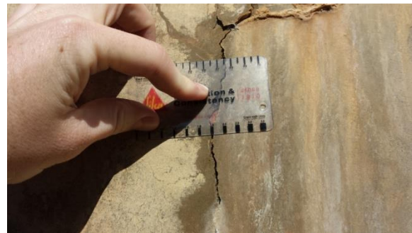
Figure 4-7: Hartbeeskuil Dam: Crack width and typical ASR crack staining
