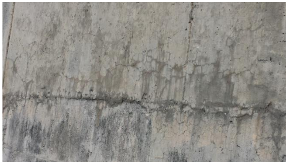
Figure 5-6: Poortjieskloof Dam: Some more map cracking on the concrete step structure
