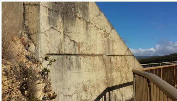
Figure 4-6: Hartbeeskuil Dam: AAR cracking pattern on the far-right abutment steps
