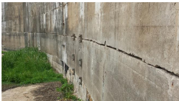
Figure 5-14: Poortjieskloof Dam: Clear separation of first horizontal construction lift joint above apron
