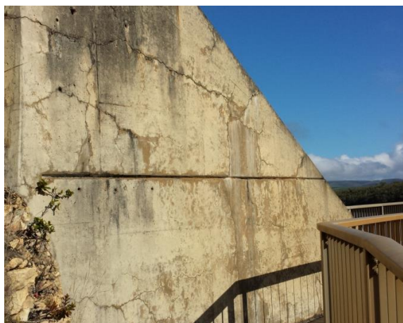
Figure 2-1: Typical ASR crack pattern and staining
