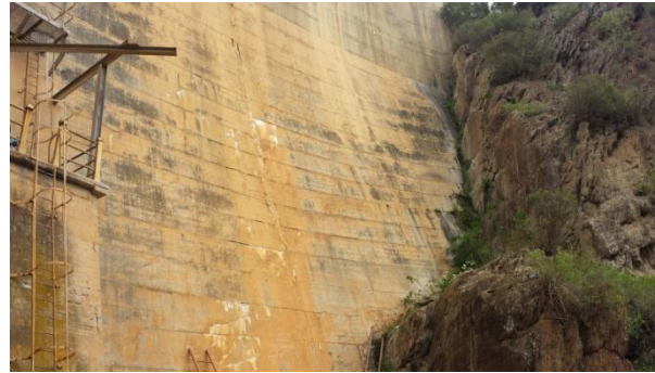
Figure 2-15: Typical peripheral cracks at Poortjieskloof Dam in South Africa
