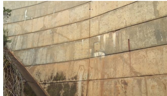
Figure 4-11: Hartebeeskuil Dam: Parallel cracks in the vicinity of the "pulvino"
