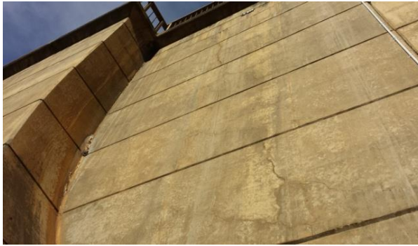
Figure 4-8: Hartebeeskuil Dam: Typical parallel peripheral cracks in the vicinity of the right flank "pulvino"
