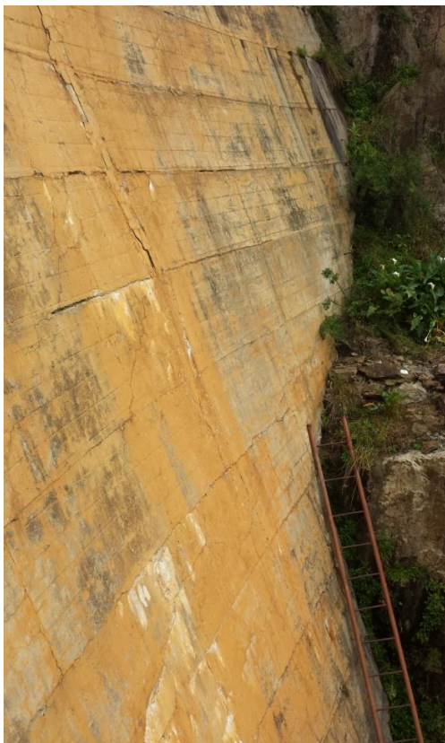
Figure 5-9: Poortjieskloof Dam: Some seepage through horizontal lift joints bordering the left abutment
