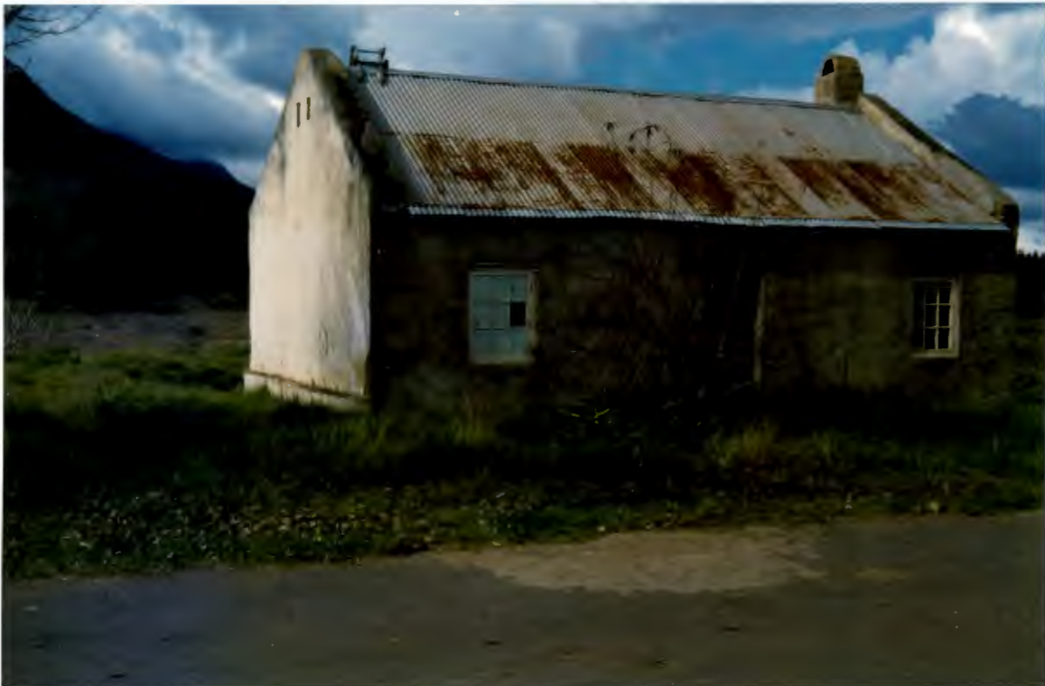
The end of the road - no longer productive since forced removal of the tenant - and awaiting renovation.
