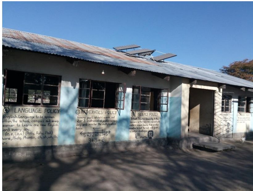
Figure 6.10: Solar panel installed at the class room block, Source: Author, 2018
