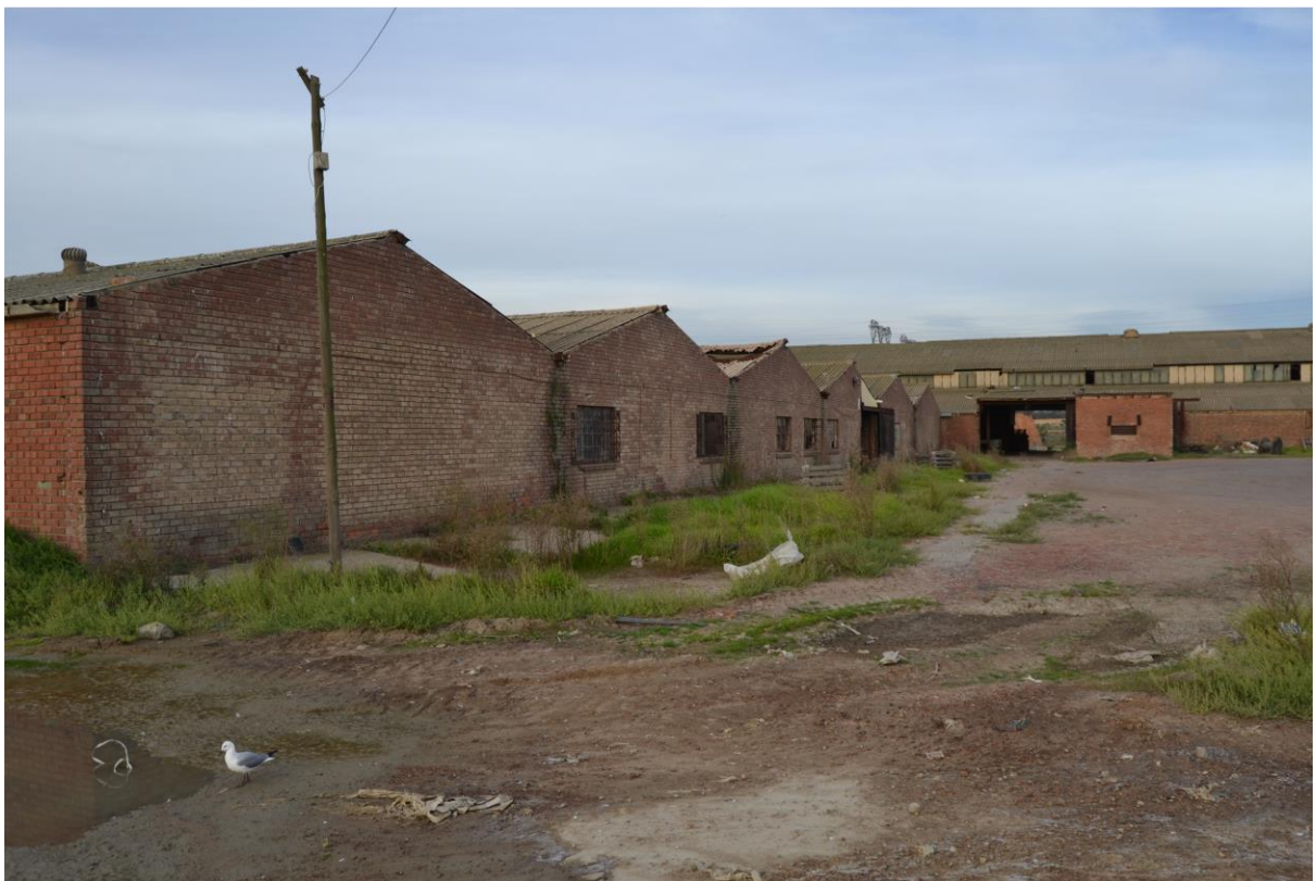
Figure 22: Image showing external area of western and southern façade of the existing building (Author, 2023).
