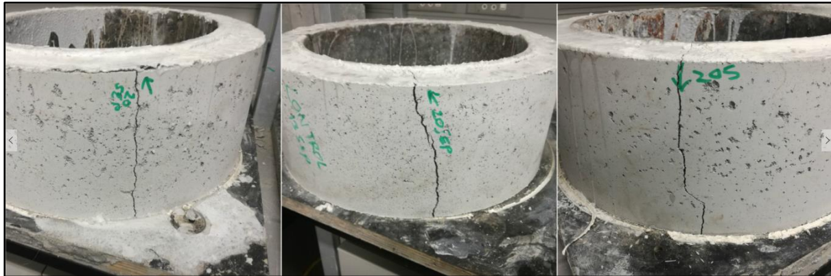
Figure 4-47: Crack distribution on control rings
