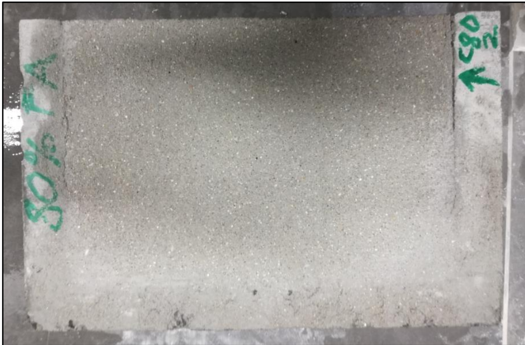
Figure 4-16: 80% FA patch repair after cyclic wetting and drying
