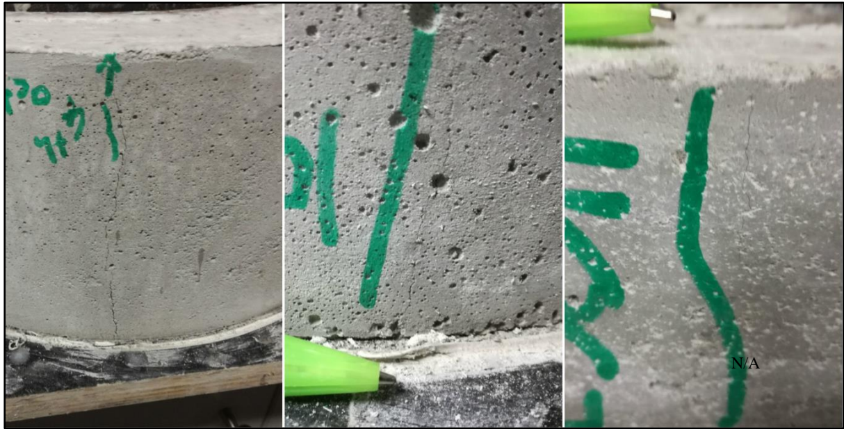
Figure 4-44: Crack distribution on 100% FA rings
