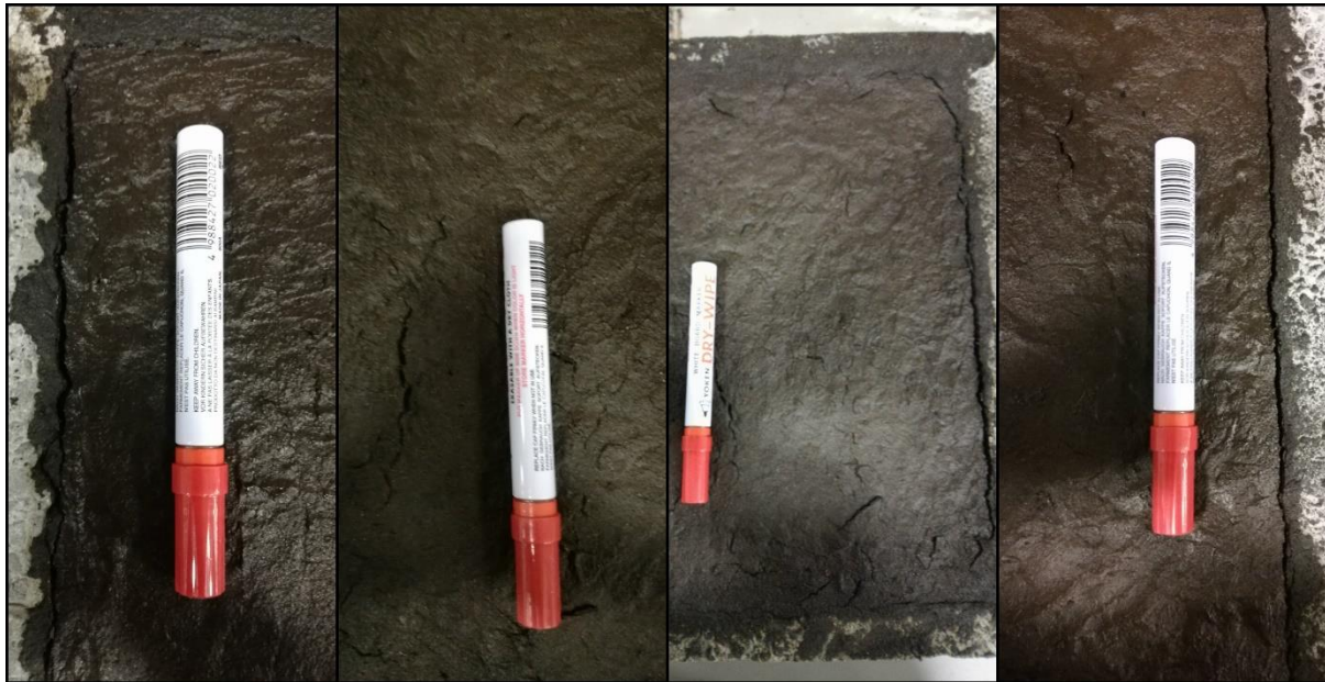
Figure 4-2: Excessive cracking and debonding occurrence on bitumen patch repairs
