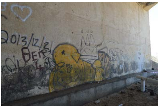
(c) Cracked abutment wall
