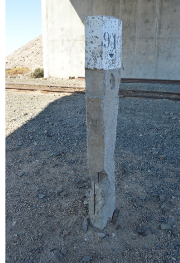
(b) Cracked rail marker
