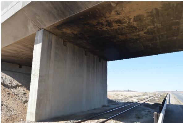
(b) smoke stained deck soffit
