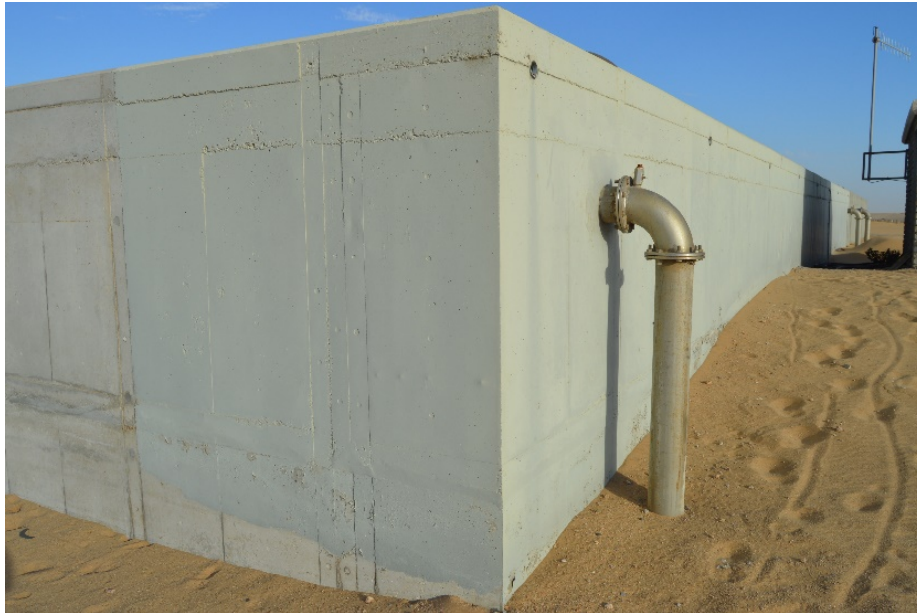
Fig. 6-12: Aphrodite beach water tank
