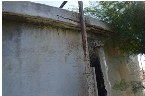
(b) Cracked roof slab edge
