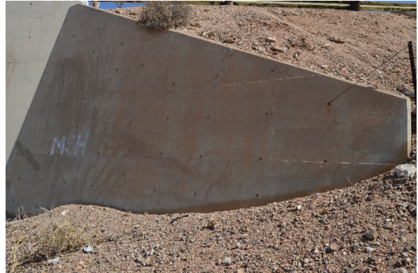
(c) Wingwall with a diagonal crack
