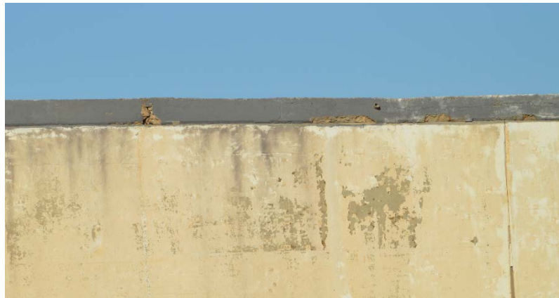
(c) Corrosion damage on tank roof slab
