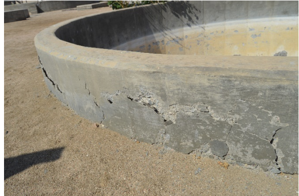
(b) cracked empty water treatment pond
