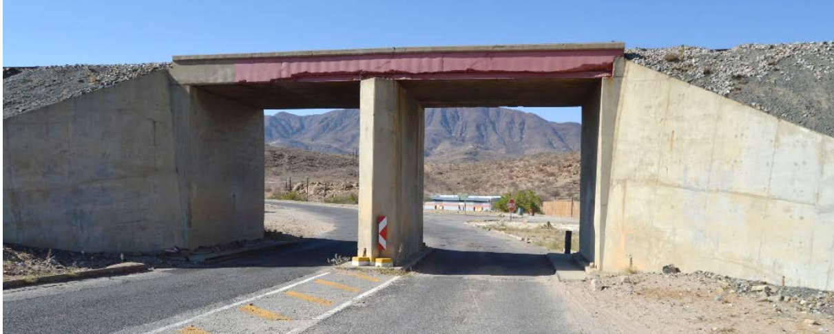
(a) Usakos Rail over road bridge with chipped parapet foot
