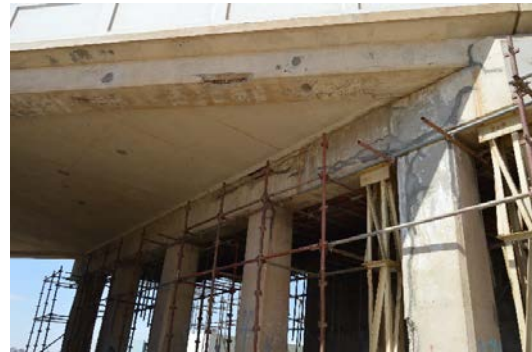
(b) Cracked bridge beam
