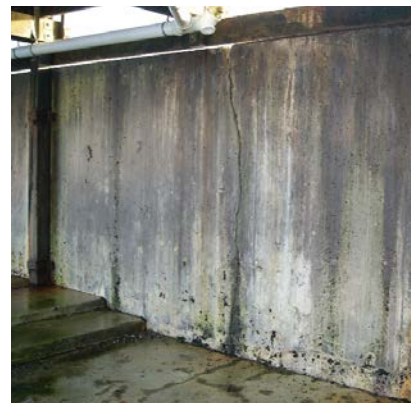
(b) Vertical crack in retaining wall
