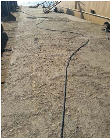
(e) Surface material loss
