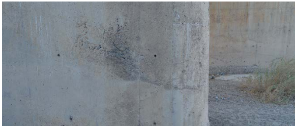
(c) Honeycombed pier wall
