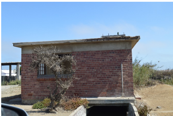
(e) Cracked pump house roof
