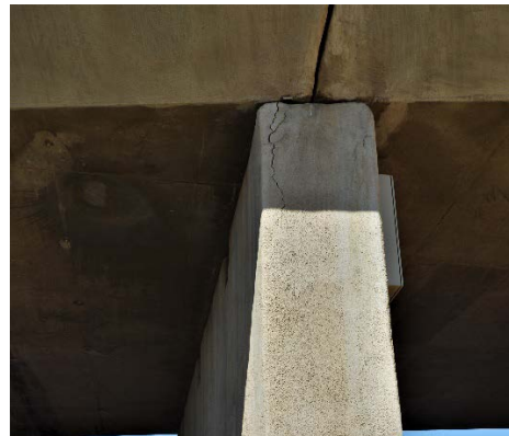
(c) Cracked pier top
