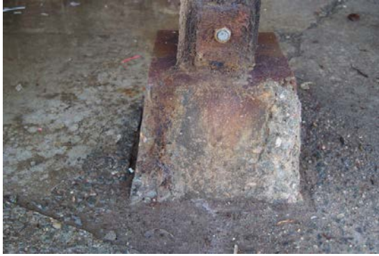
(c) Stub column cracking
