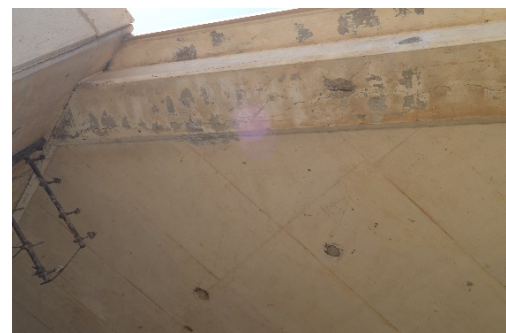
(g) Cracked beam
