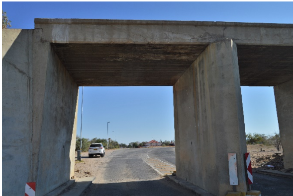
(b) Deck damaged
