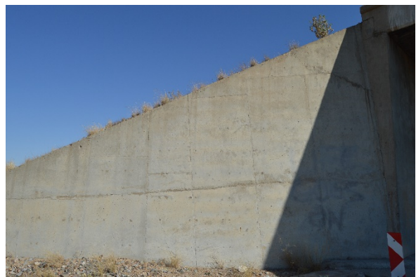
(c) Wingwall with diagonal cracks
