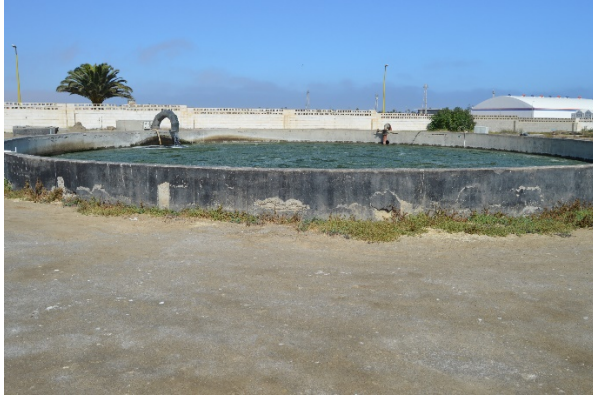
(a) cracked pond with wastewater
