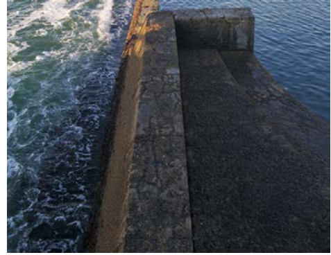
(d) Breakwater having surface concrete material loss, cracking and delamination
