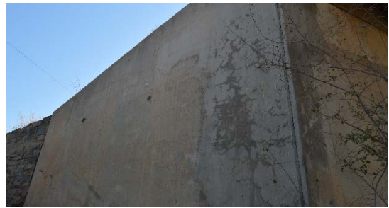
(b) Patched wingwall with cracks
