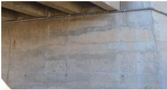
(b) Vertical crack on abutment wall
