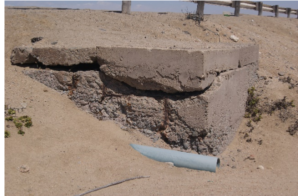
(c) Water manhole with concrete delamination
