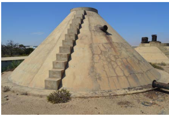
(c) Cracked digester roof
