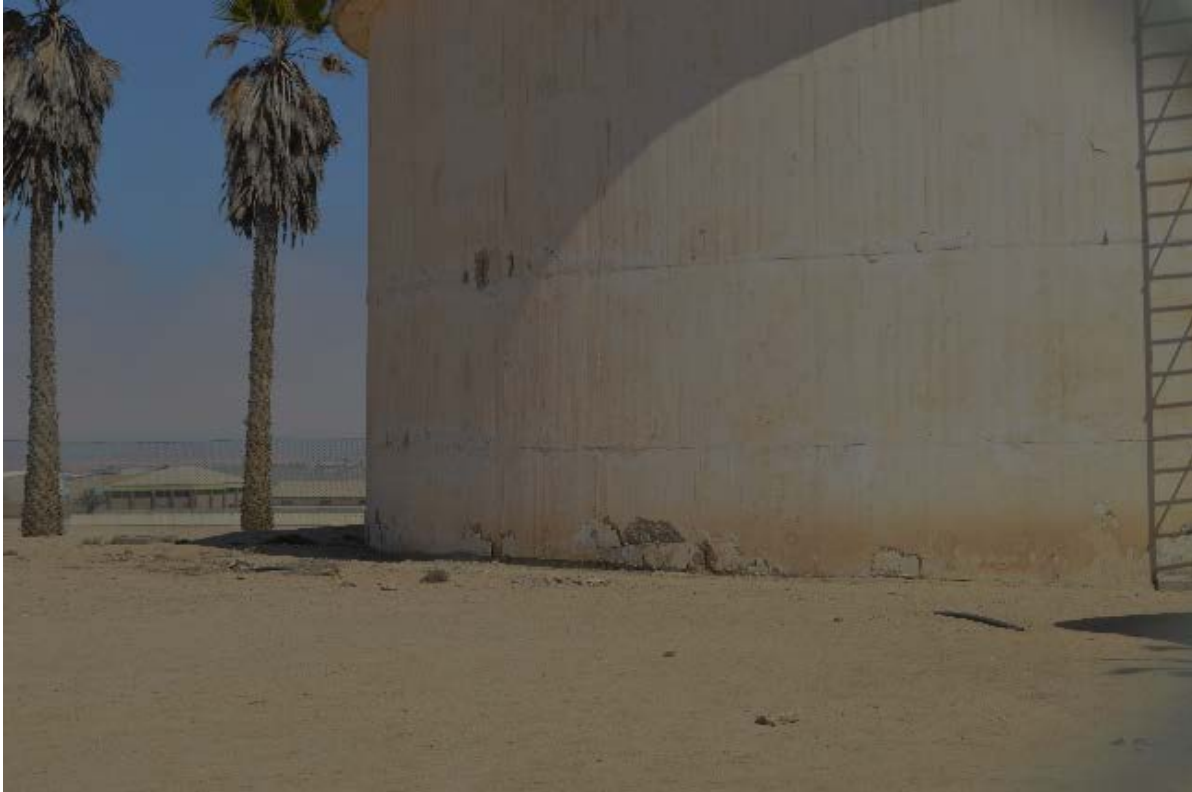
Fig. 6-15: showing concrete defects on Mondesa tank
