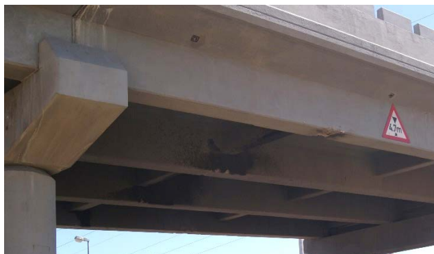
(a) Impact damage to bridge soffit
