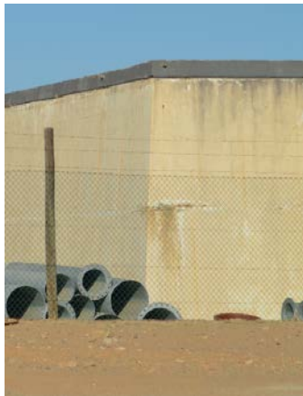
(b) mid-height leakage
