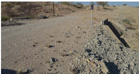
(e) Cracked headwall
