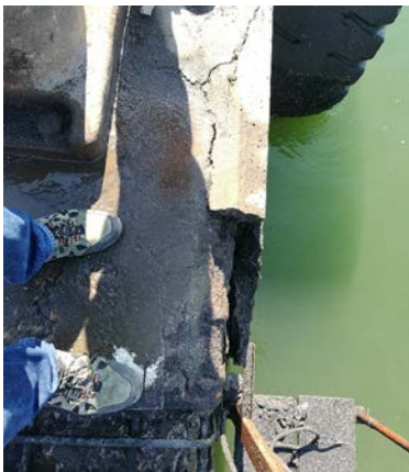
(a) Concrete spalling
