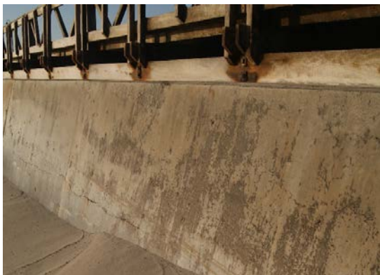
(a) Cracked concrete retaining wall
