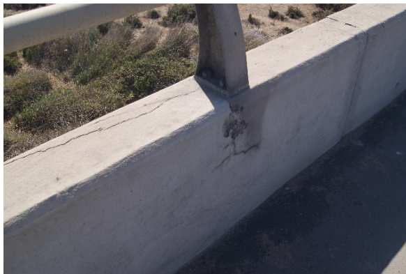
(b) Cracked parapet upstand beam
