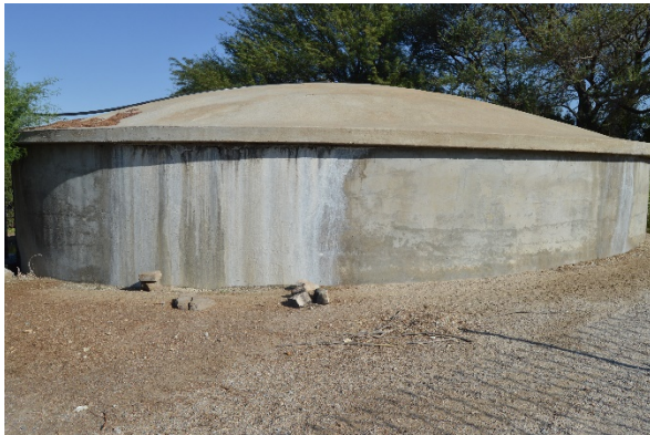
(a) Off-B2 water tank
