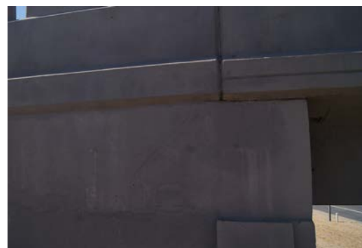
(b) Abutment with a diagonal crack
