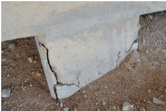
(c) Crashed abutment
