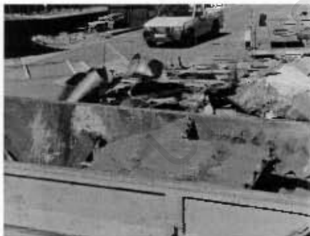
Figure A.3: Demolished steel sorted for recycling, South Africa Source: Irurah (1999) cited in Irurah (2002)
