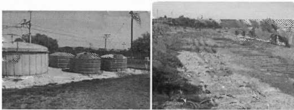
Figure 9: Biolytic Tanks and the surface area of the vertically constructed wetland -Lynedoch Eco Village
