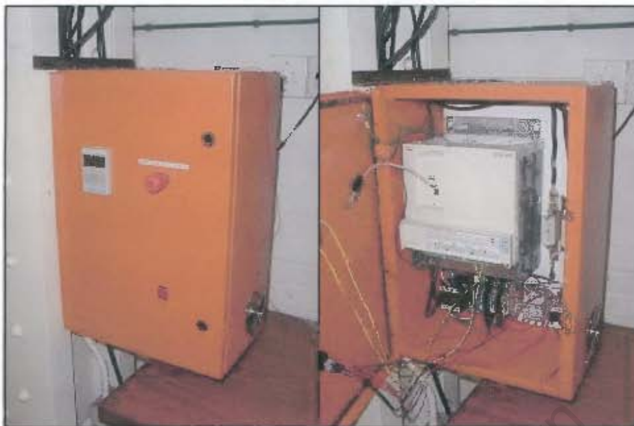
Figure A-7 The new DC Drive used for dynamometer control.
