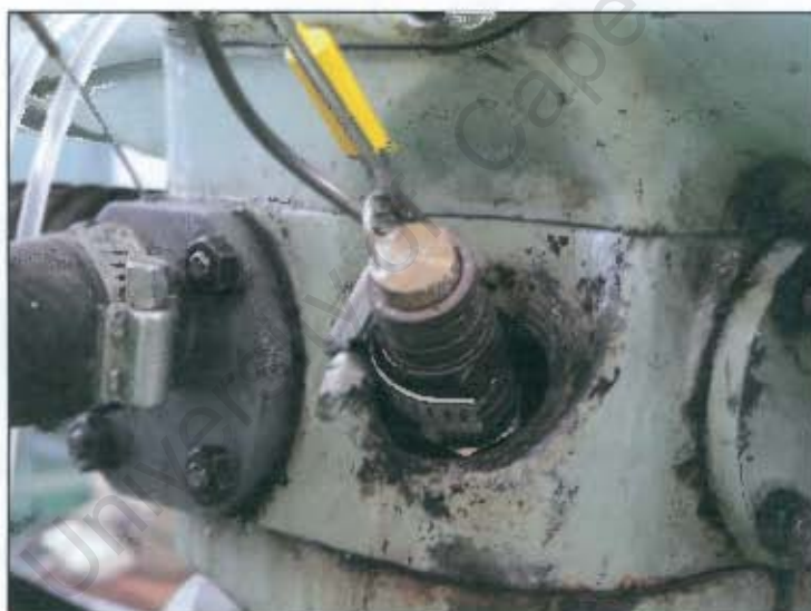
Figure 4-6 The Hot Tube igniter installed on the engine.
