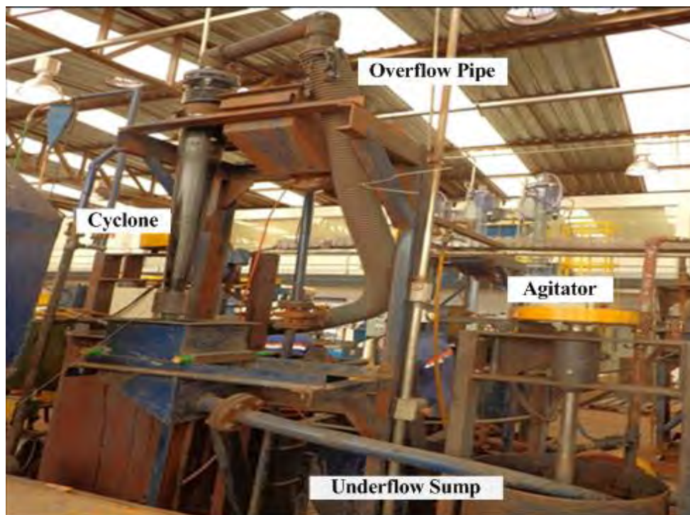
Figure 3-2: Picture showing the Anglo American hydrocyclone rig
