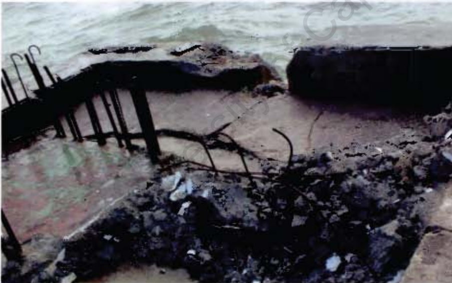
Figure 5-8: Settled Slab at Lighthouse end of Eastern Breakwater
