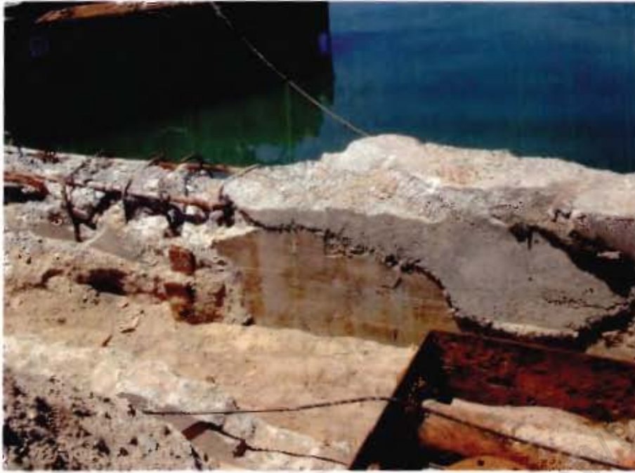
Figure 5-17: Previously performed patch repairs
