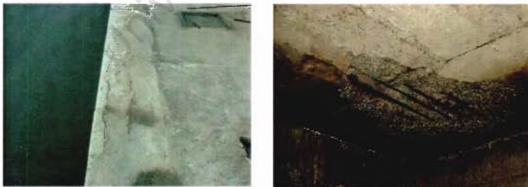
Figure 2-8: Concrete deteriorated due to cracking and spalling (Source: Author)
