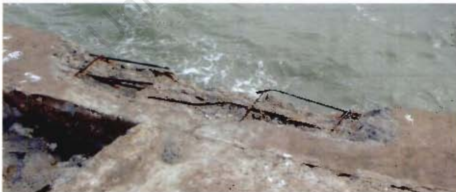
Figure 5-2: Spalling to Western Breakwater (Typical across site)
