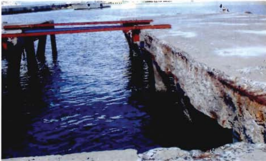
Figure 5-14: Collapsed bay of Turning Mole, showing damaged steel reinforcement
