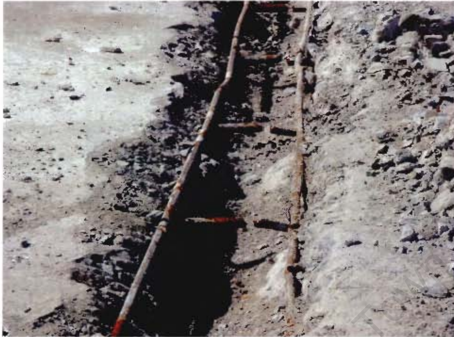
Figure 5-11: General Corrosion damage
