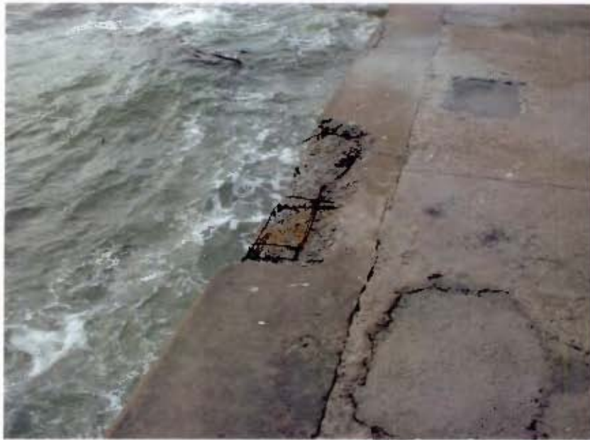
Figure 5-4: Spalling to Edge Beam
