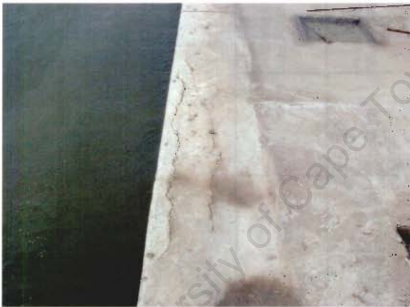
Figure 5-3: Cracking to Edge Beam
