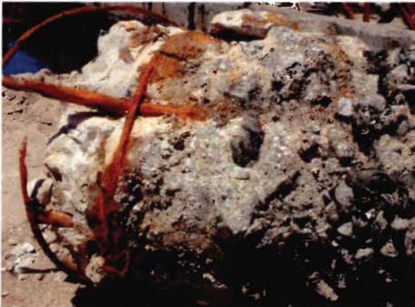
Figure 5-20: Severe damage to Trawler Quay beams and columns
