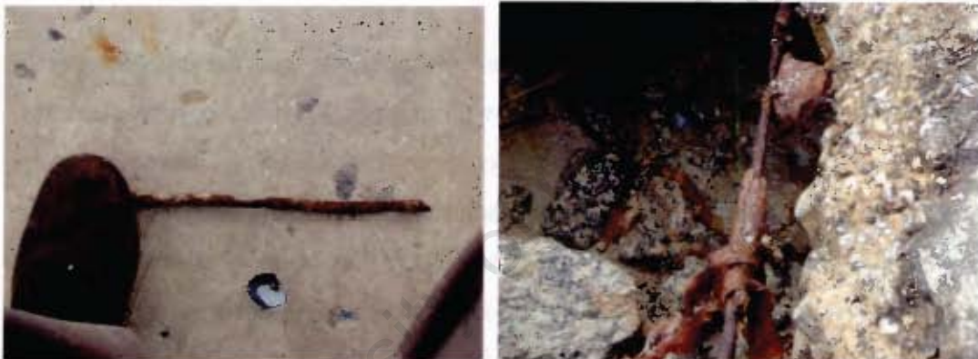
Figure 5-5: Severe loss of section due to corrosion
