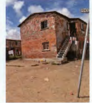
Figure 42: Loose sandy soil
