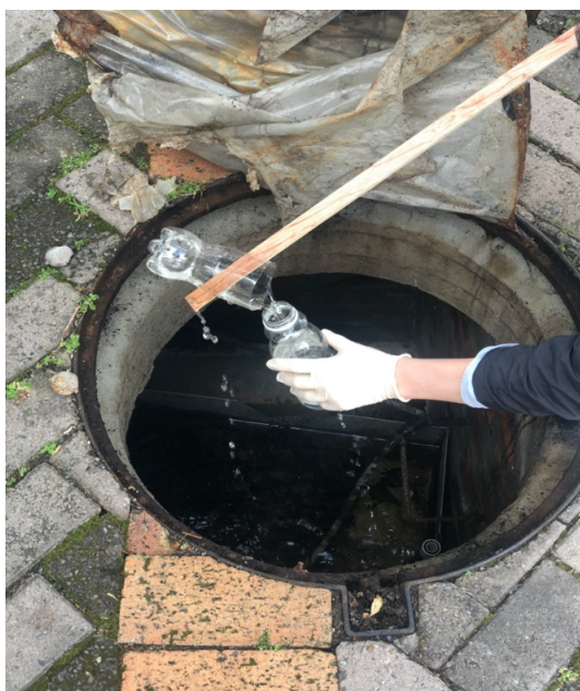
Figure 3-37: Using a simple experiment (bottle attached with stick) to collect water from the monitoring chamber
