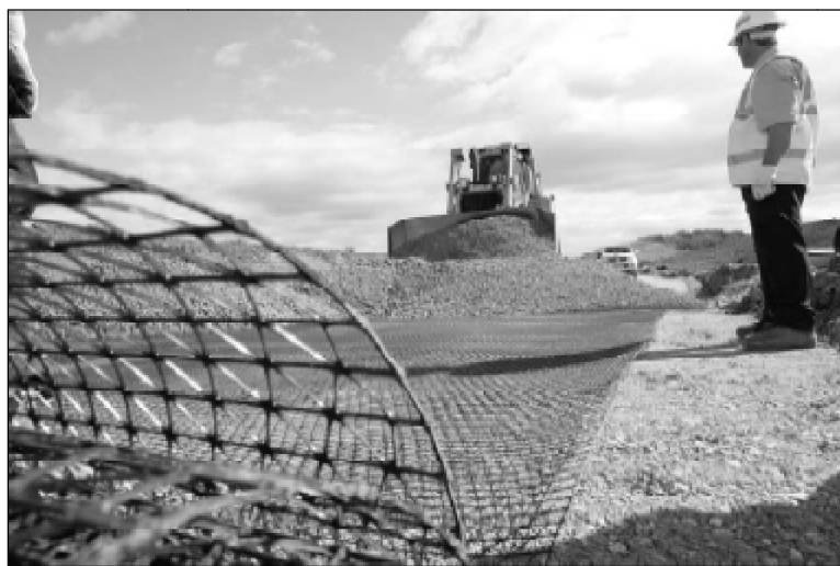
Figure 2.6: Application of a geogrid in the sub-base during the construction of a highway across a marsh area (Tensar, 2008)
