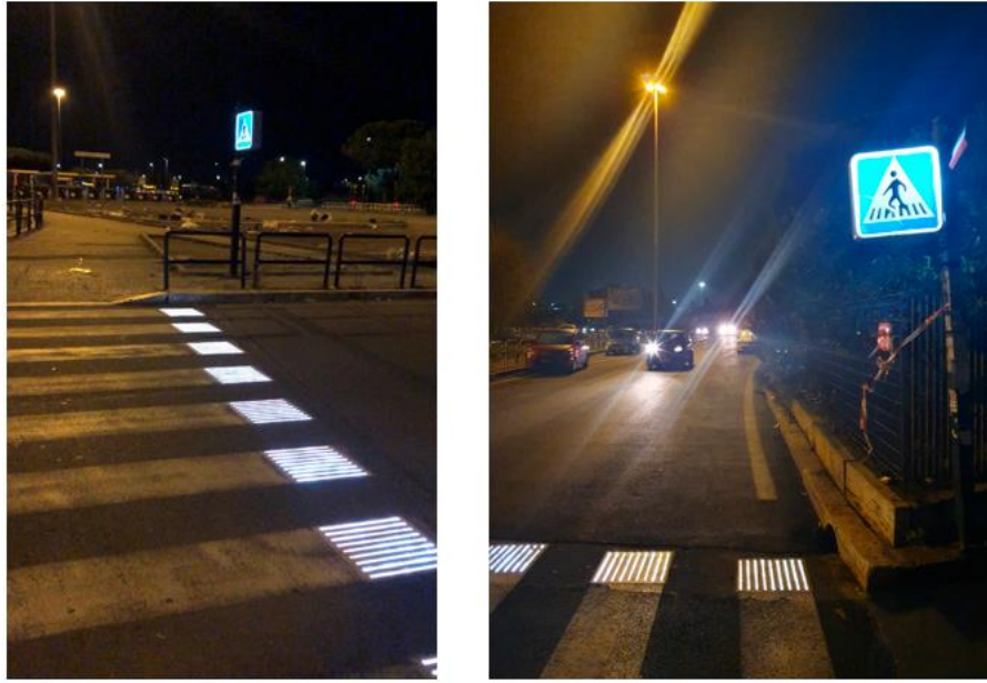
Figure 29: LED Crosswalk lighting system (Patella, S.M, et al., 2020).
