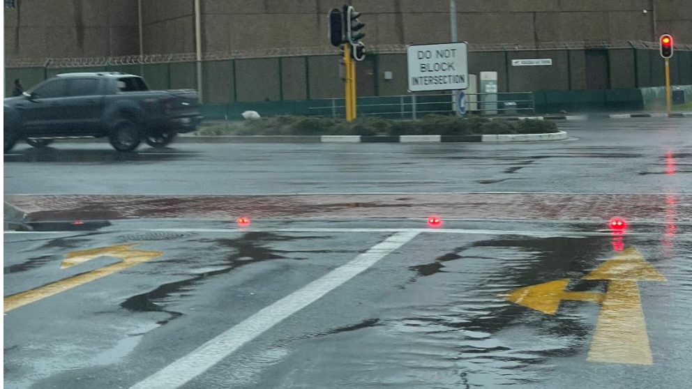
Figure 49: LED Lane Lights (Buitengracht Street outbound)
