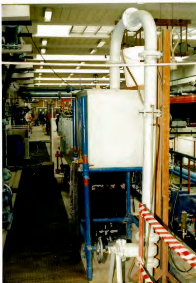
plate 4.4 : inlet valve and tank
