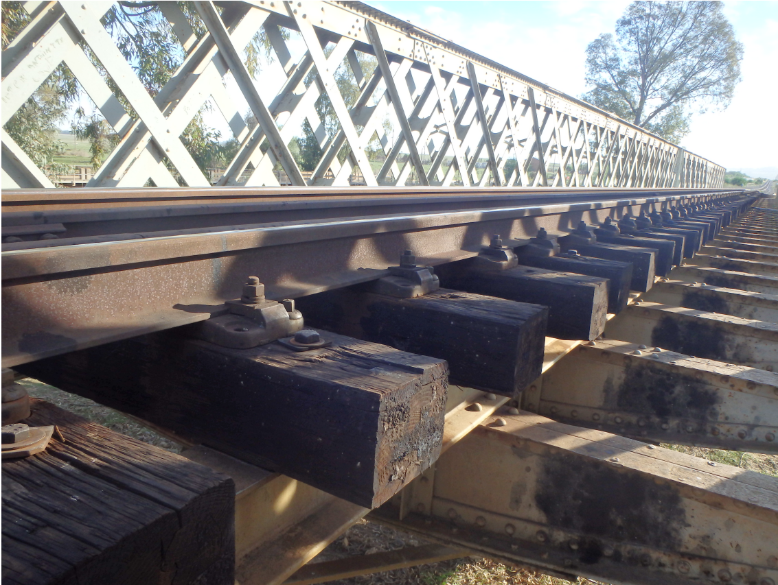
Figure 2.1: Wooden sleepers on open deck bridge bridge (Kalbaskraal Bridge Western Cape South Africa)
