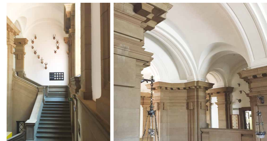
Figures 43 & 44 Sandstone stairwell leading to the Genesis of Life I exhibition hall; arched ceiling, DNMNH.
