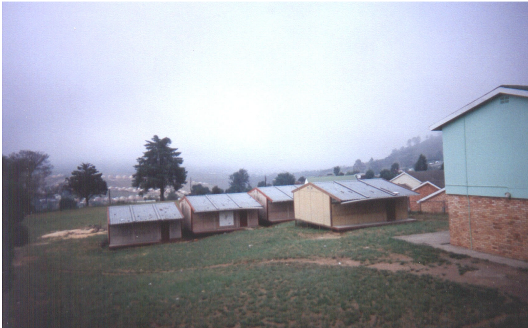
Figure 6.5 Disused Weather-Damaged Mobile Classrooms at Knysna. Note boarded up windows and collapse roofs.
