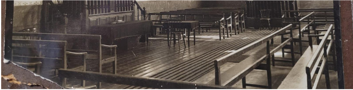
Figure 42: The wooden floors visible inside the church building. (Source: Dutch Reformed Mission Church Wellington)
