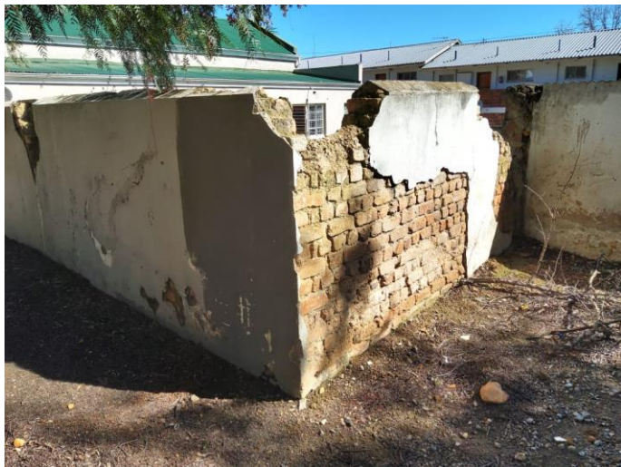
Figure 10: Raw brick and clay ring wall remnants of the church yard in poor condition. (Photo: Pierre-Jeanne Gerber, 2020)
