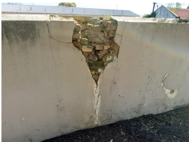
Figure 11: Damaged raw brick and clay ring wall badly joined with cement and bricks. (Photo: Pierre-Jeanne Gerber, 2020)
