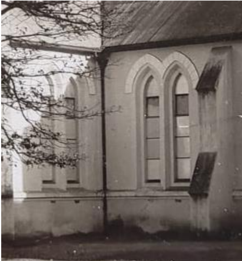
Figure 37: Indicating the gutters and downpipes on the side of the building. (Source: Dutch Reformed Mission Church Wellington)
