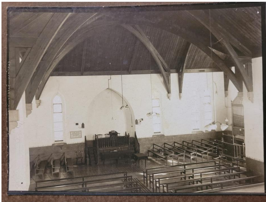
Figure 36: This photograph shows the hammerbeam roof trusses resting on granite or stone corbels, and the Oregon pine tongue-and-groove ceiling. (Source: Dutch Reformed Mission Church Wellington)
