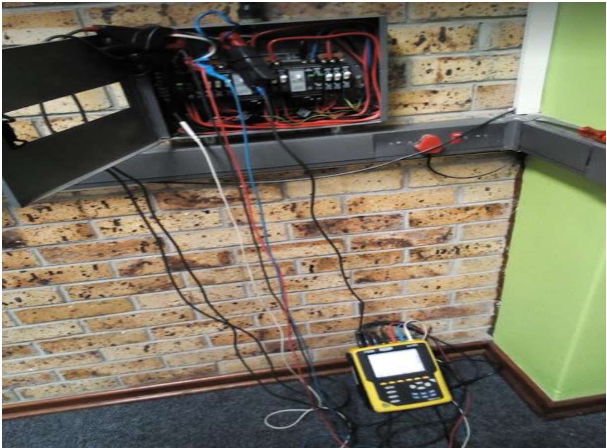
Figure 6-10: Practical Connection PQ Analyzer for the Measurement
