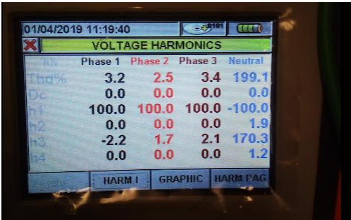
Figure 6-11: Voltage harmonics of the computer laboratory
