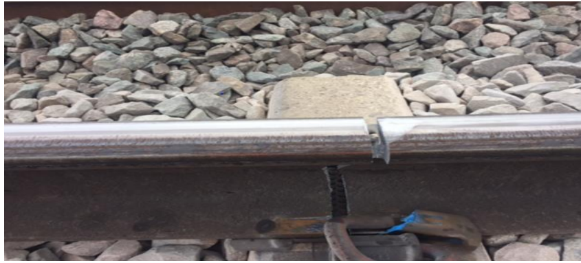
Figure 2.11: Broken rail (Network Rail, 2021)
