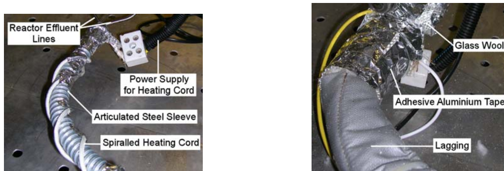
(a) Uninsulated product line immediately preceding vaporisers
