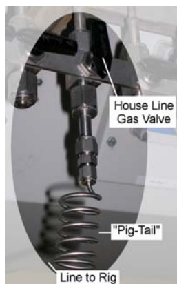
(a) Tubing formed into a "pig-tail" and attached to house line valve manifold
