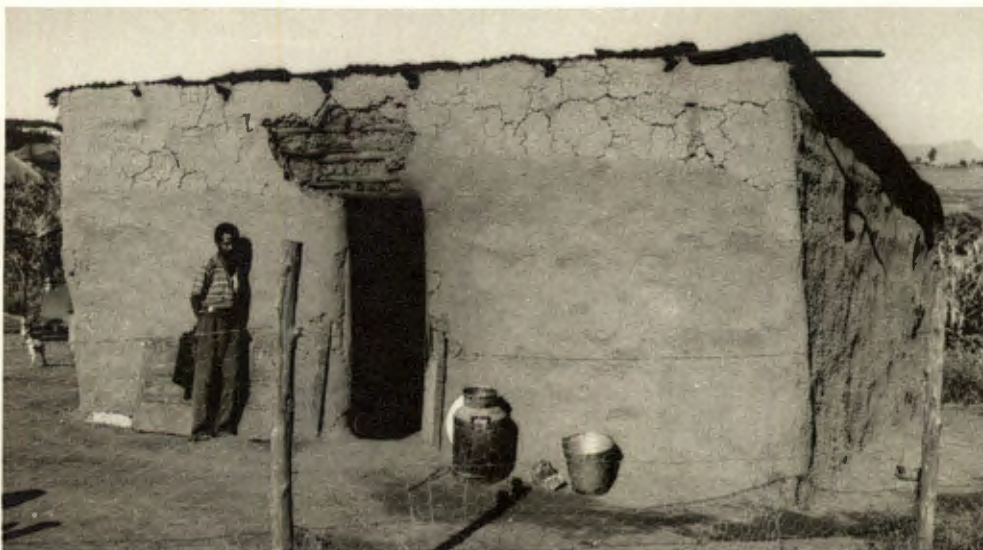
The home of Thabethe Co.No.2064/217 at Howick West. There are 4 rooms 10' x 8': back wall 5' high: front wall 7' high. No chimney, and the hearth is in the centre of the diningroom floor. Small window apertures 14" x 14" are provided in the bedrooms.
