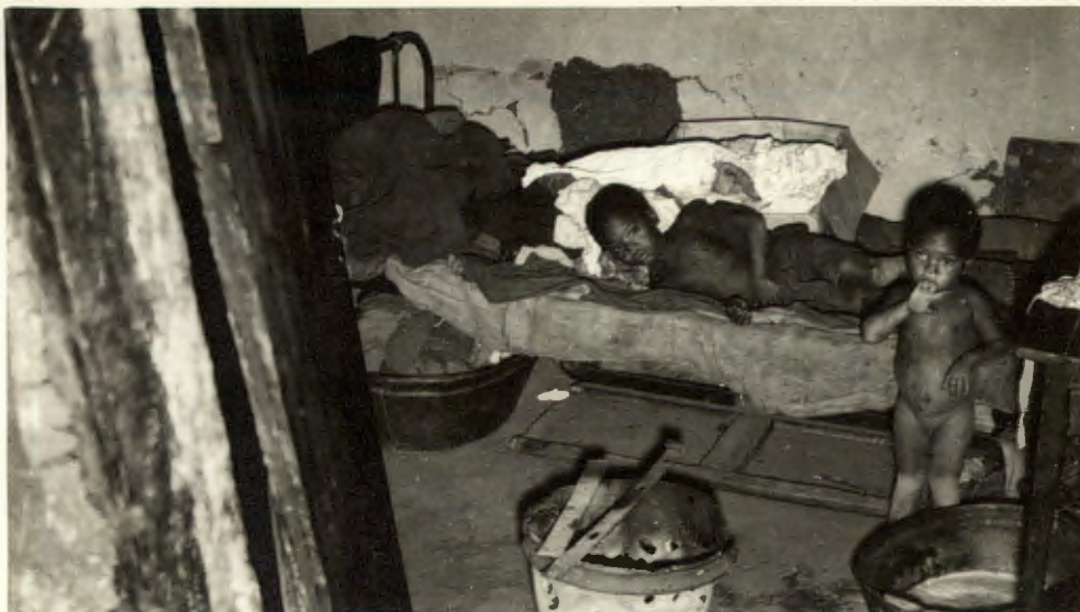
In this room of Ronald Maseko's house cooking is done on the brazier in the foreground. The angle of the door joint is shown at the left foreground, evidence of the condition of the house which leans over and soon may become dangerous.
