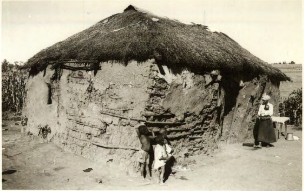
The home of Ronald Maseko Co. No. 6457/209. He occupies 2 rooms and has lodgers in the three remaining rooms. This is one of the worst shacks in Howick West. It is in a very poor state of repair and patches of sky are visible through the roof.
