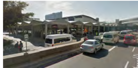
fig.60 - The existing roof over Ticket Hall on Strand Street. (source: Google Street View)
