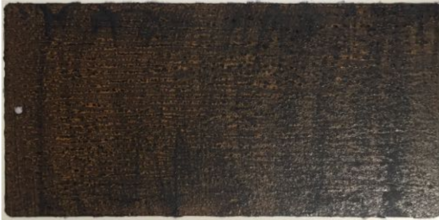
Figure 6: Sample with no salt contamination and chemical (rust converter) surface preparation (NC1) prior coating application
